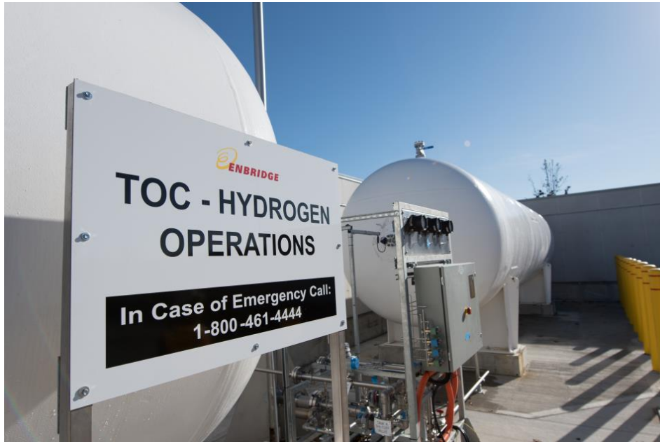
Figure 3: Enbridge Hydrogen Storage Tanks
