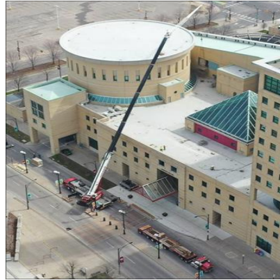
Mississauga City Hall Mechanical Replacement
