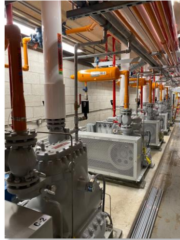
New Refrigeration Plant
