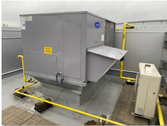
New Roof Top Unit
