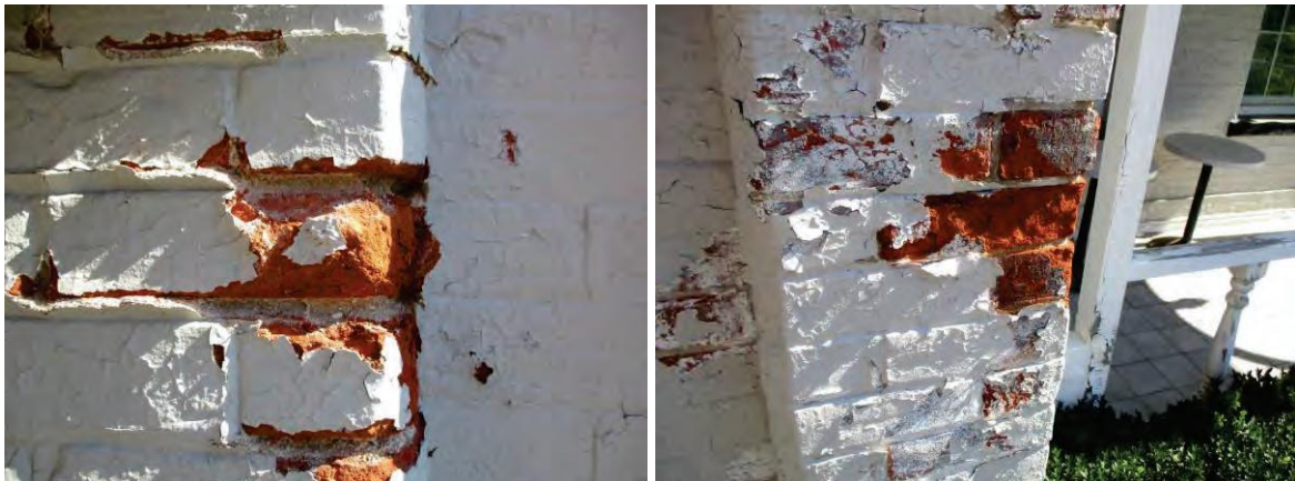
Figure 6a, 6b: Damage to masonry at south side of entry canopy
