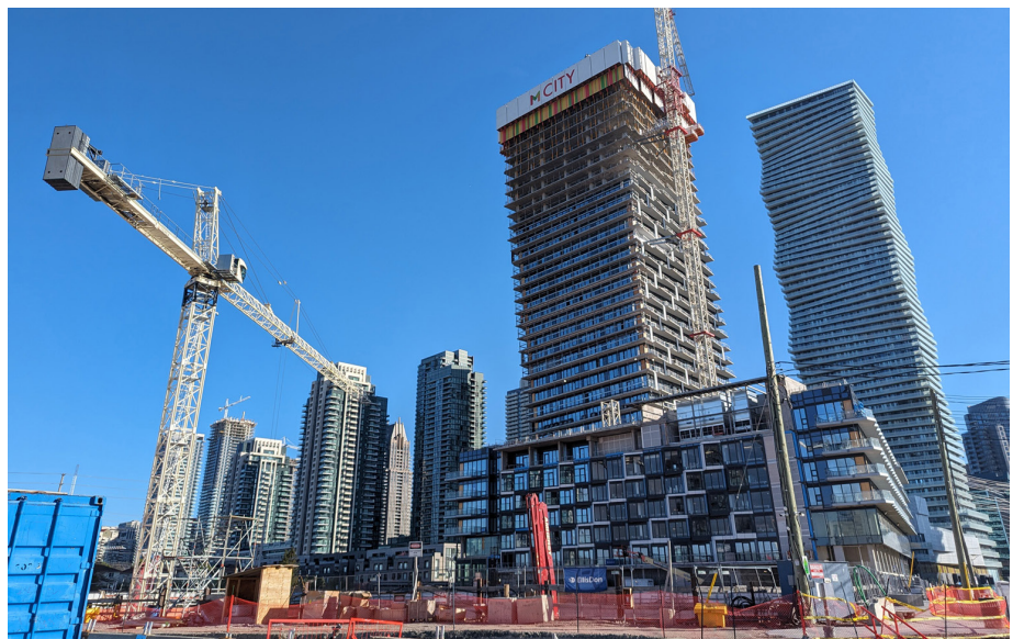
A condo building being constructed in Mississauga's downtown core. Photo: City of Mississauga
