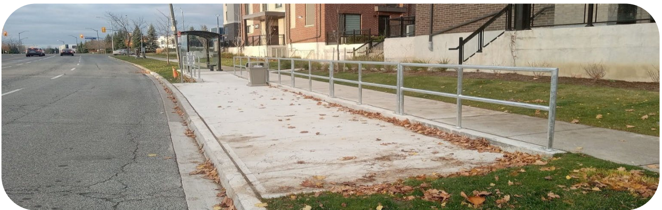
Figure 2: Landing pad with ramp connection at bus stop#0527 The Collegeway at Ridgeway Dr. that meets the slope requirements.
