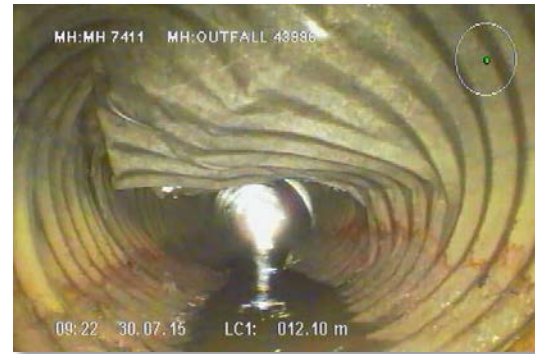
Aging stormwater infrastructure
