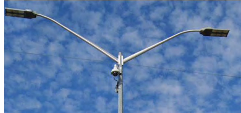
CCTV Camera mounted on Street Light Pole
