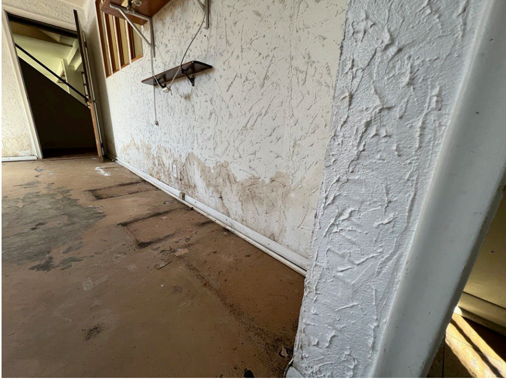
BASEMENT SHOWING WATER STAINING, MOULD
