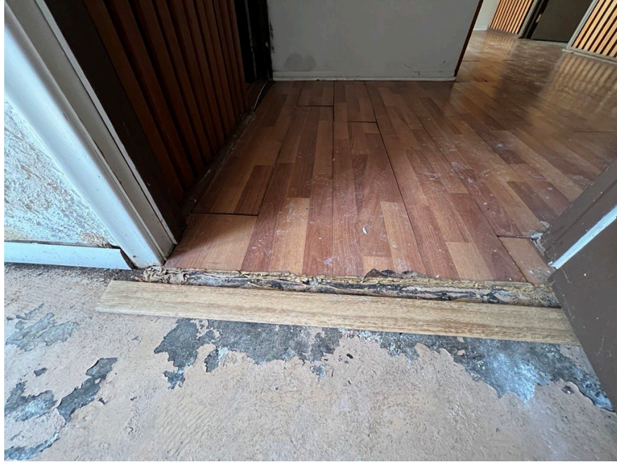
TYPICAL BASEMENT FLOOR. NOTE ENGINEERED WOOD FLOOR DAMAGED FROM FLOODING
