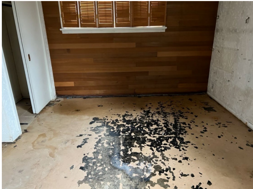
WATER STAINING AND STANDING WATER ON THE BASEMENT FLOOR. WATER APPEARS TO BE COMING FROM DAMAGED AREA AT RIGHT
