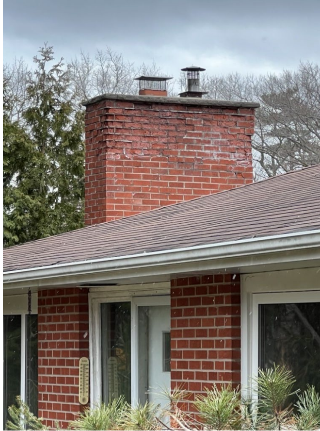
BRICK CHIMNEY DETERIORATION
