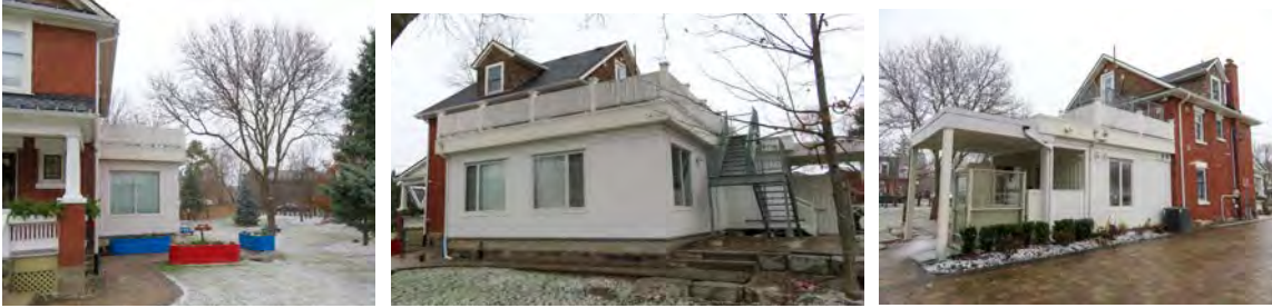
REAR ADDITION - the existing 1-storey rear addition built by Rotherglen School in 2019 is to be demolished
