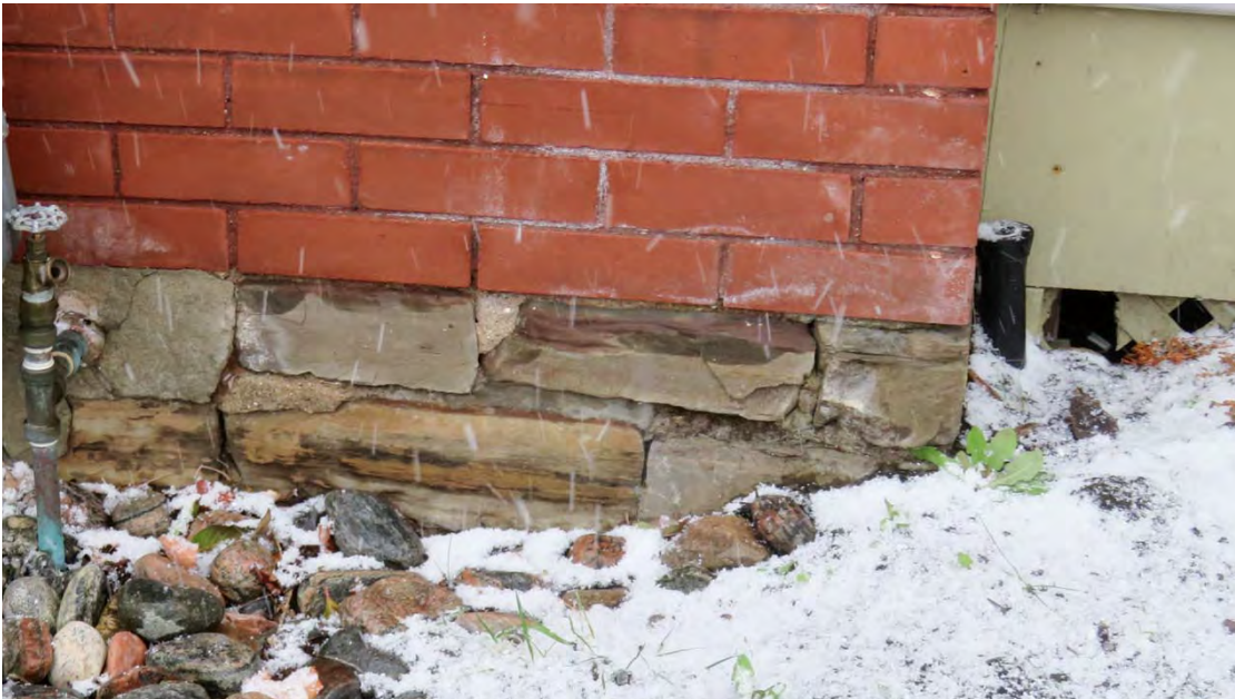
FOUNDATION – rubble foundation with credit valley stone and lime mortar – open joints and missing mortar in some locations
