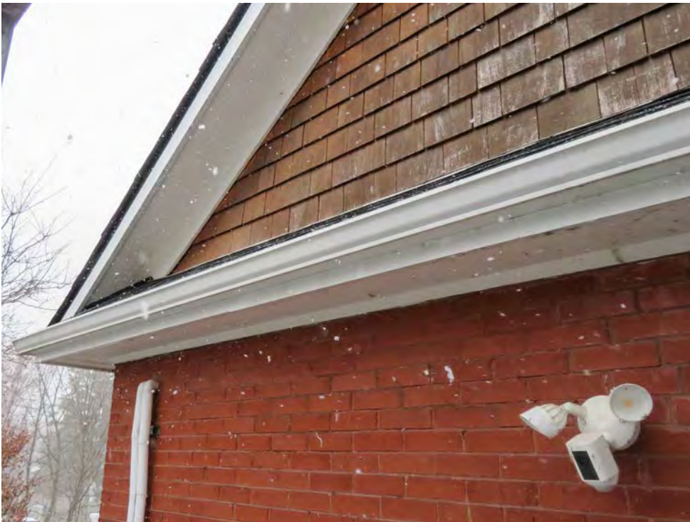
REAR ELEVATION – soffits at the rear will be removed to accommodate connection with the new addition – the wood shingle in the gable is not original
