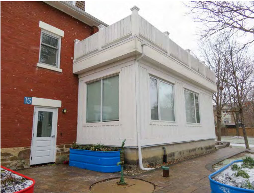
REAR ADDITION – TO BE DEMOLISHED – non-historic addition to be demolished – wraps around the back corner of the building – it has a concrete block foundation and is frame construction with aluminum windows
