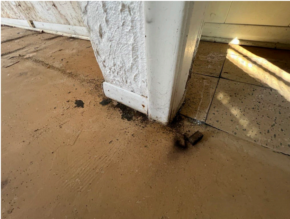
BASEMENT FLOOR WATER DAMAGE
