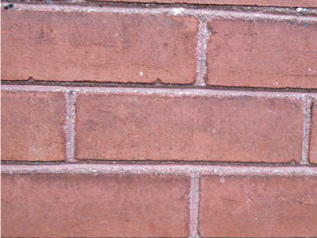
RED BRICK MASONRY – grooved mortar joint with red mortar – may have originally been tuck pointed
