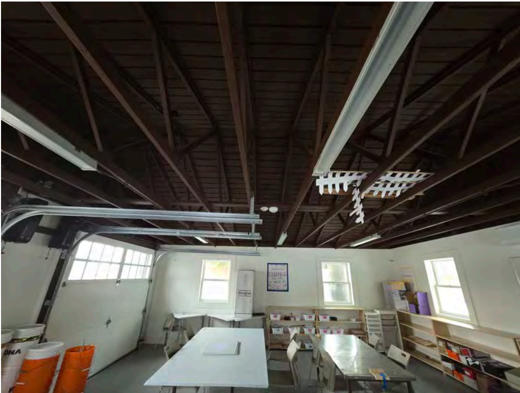
GARAGE – TO BE DEMOLISHED – a modern structure that has no cultural heritage value - concrete pad foundation – exposed roof rafters are modern dimensioned lumber – interior walls are drywall - date of construction estimated to be c.1970s or 1980s
