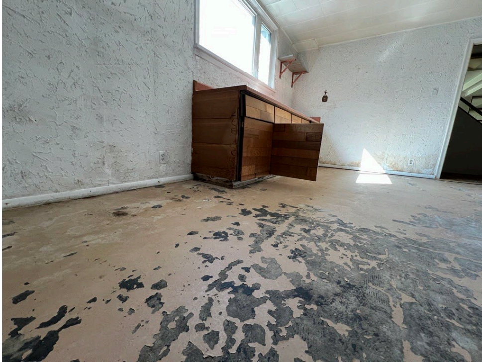
BASEMENT CABINETRY WATER DAMAGED
