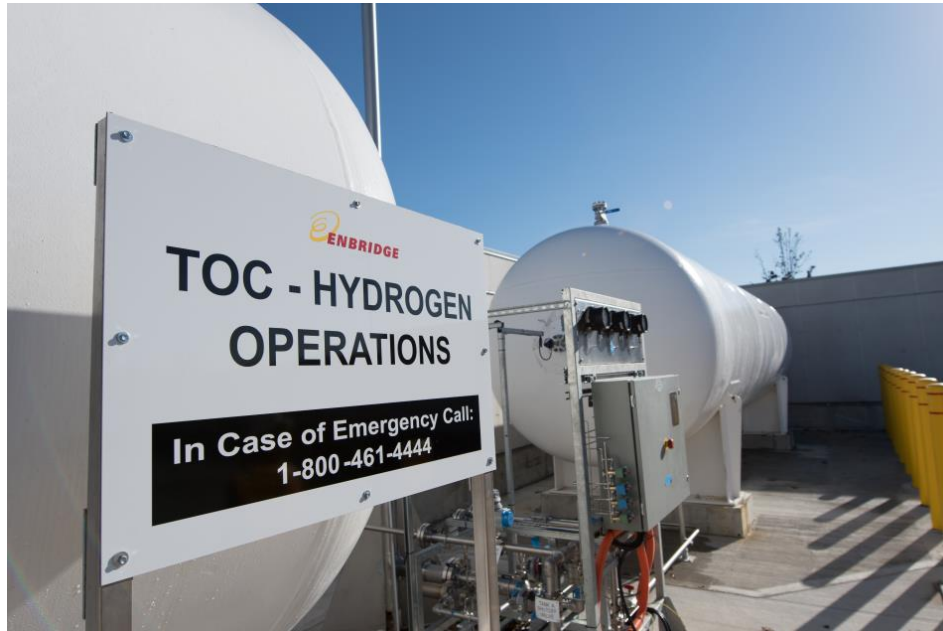
Figure 3: Enbridge Hydrogen Storage Tanks
