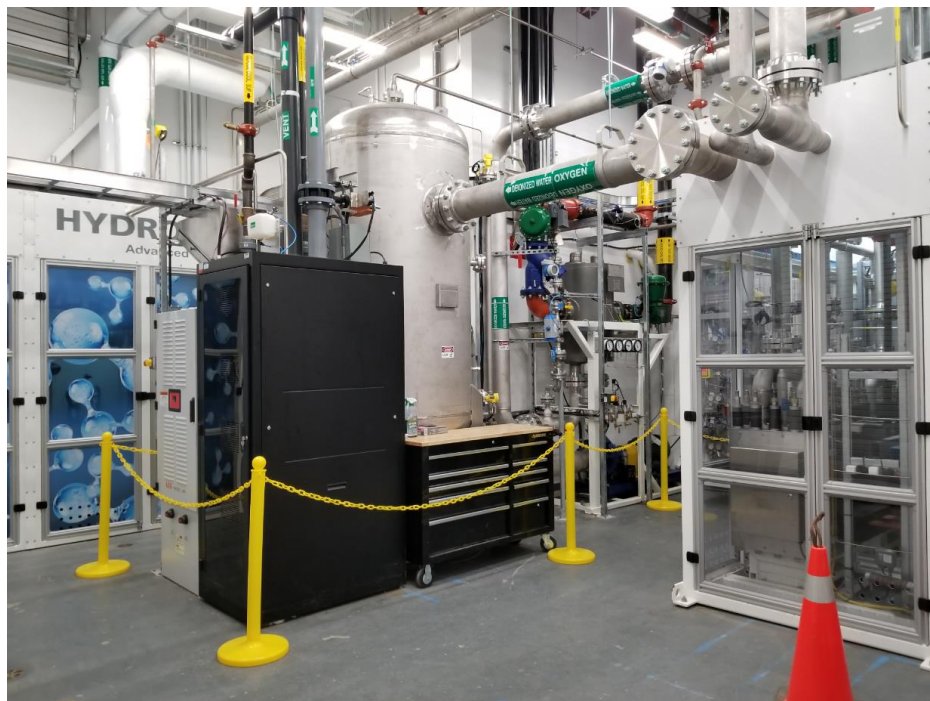
Figure 4: On-site Enbridge Hydrogen Production. Cabinet that houses the electrolyzer is shown on the right. Black box houses a fuel cell for low power lighting. Hydrogenics box contains dryer tank for final cleaning up of hydrogen.
