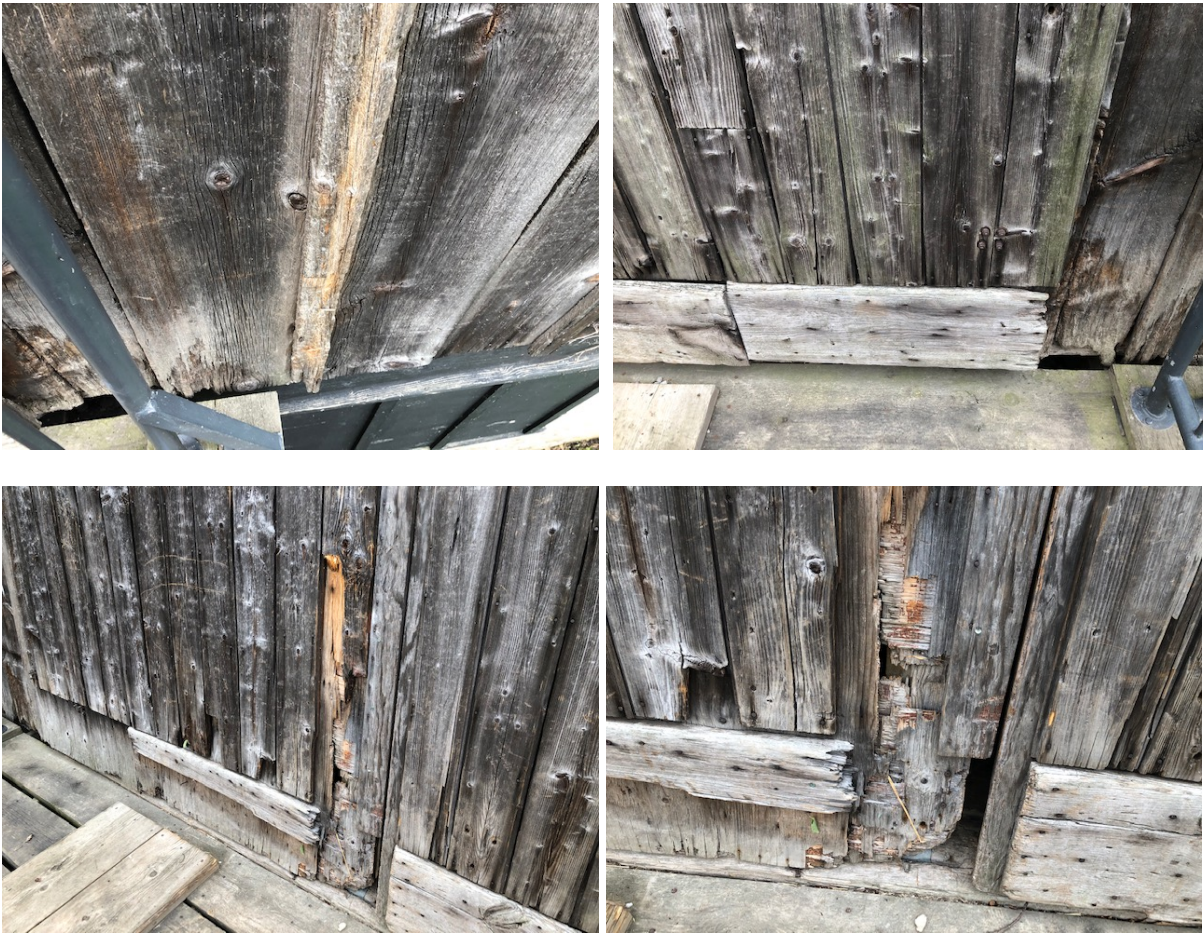
Images of typical deterioration found at the barn door located at the north elevation
