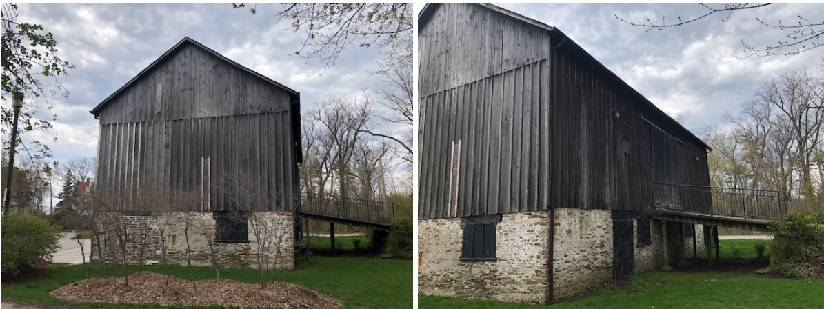
Images of typical mortar joints deterioration found
