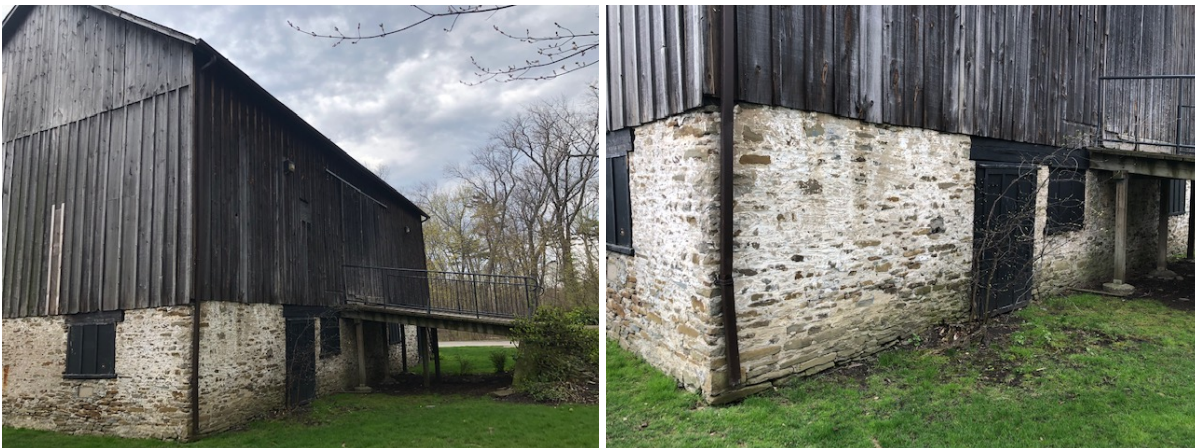
Images of typical board and batten deterioration found
