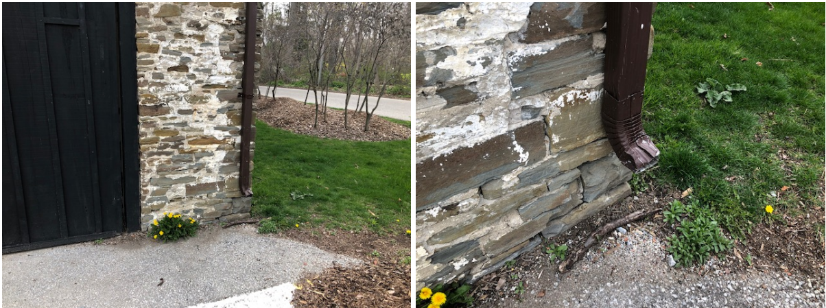
Images of typical mortar joints deterioration found at the south elevation
