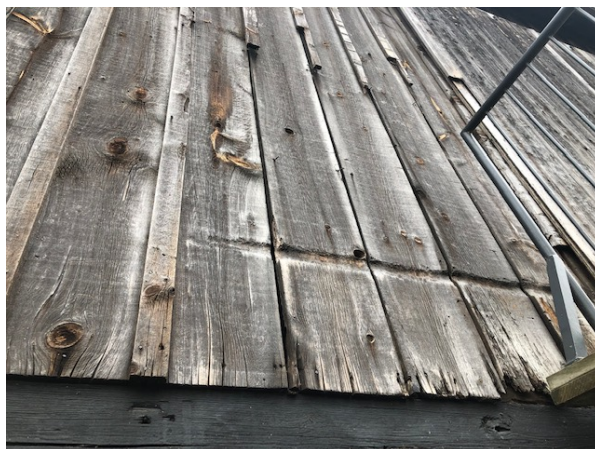
Images of typical board and batten deterioration found
