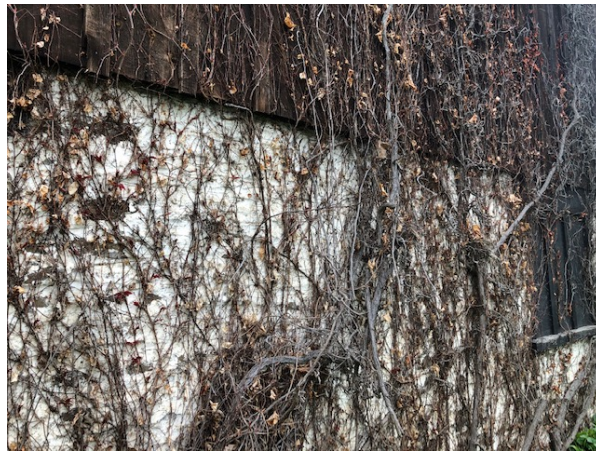
Images of typical mortar joints deterioration found at the north and west elevation
