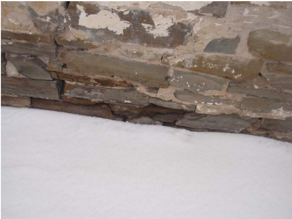
Exterior Wall To Be Re-pointed
