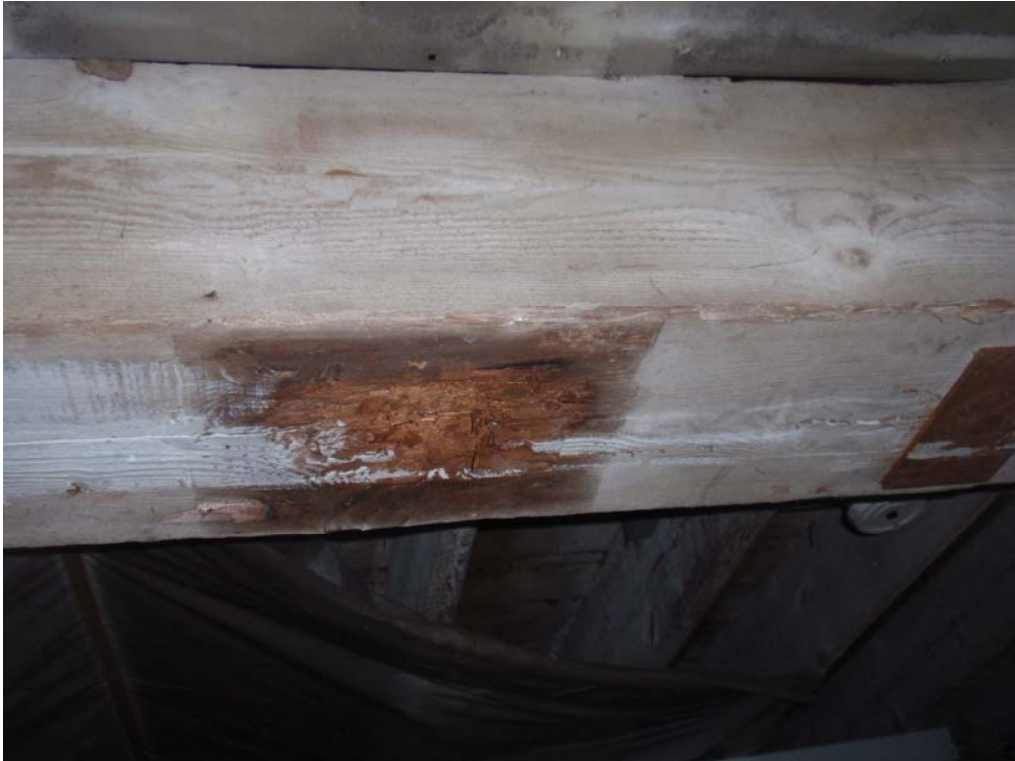
Decayed Area of Ground Floor Framing Beam
