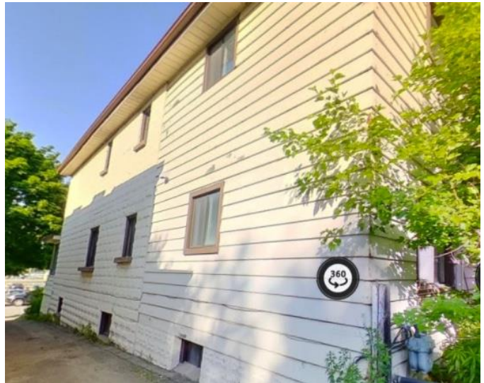
North-west side of house, part concrete block, part aluminum siding, photo Owner
