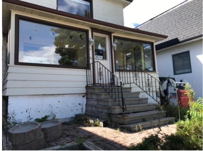
Front of enclosed porch with prefabricated concrete steps and metal railing, plate glass windows photo Picnic Design
