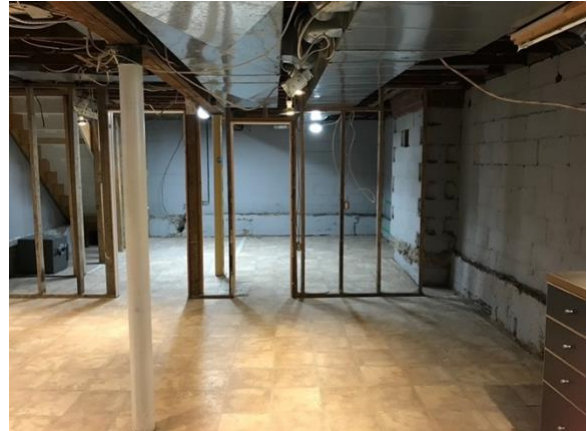
Basement, high ceilings, concrete block foundation wall has been underpinned, photo provided by owner
