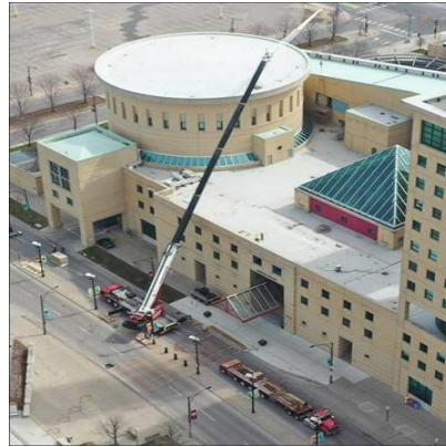
Mississauga City Hall Mechanical Replacement
