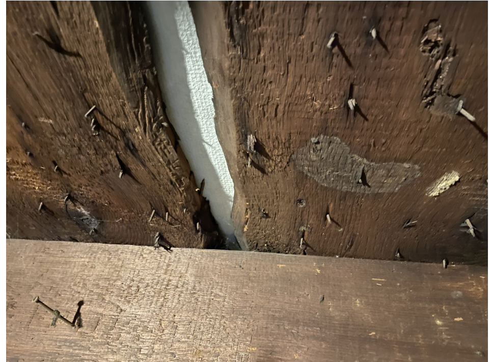
Fig. 39 Detail of the same attic's ceiling, showing an intact sheet of asbestos between boards. Note the many nail punctures in the wood.
