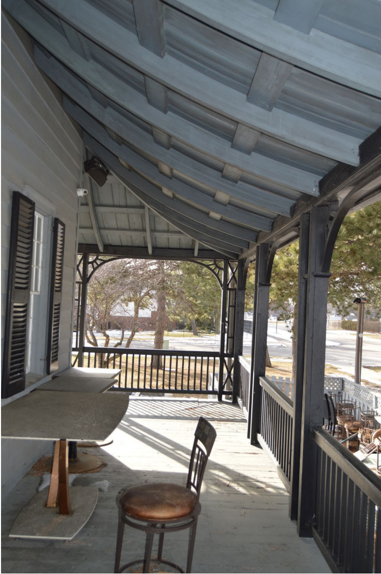
Fig. 26 Detail showing the verandah roof's wood framing in good condition. The view near the house's northwest corner looks west.
