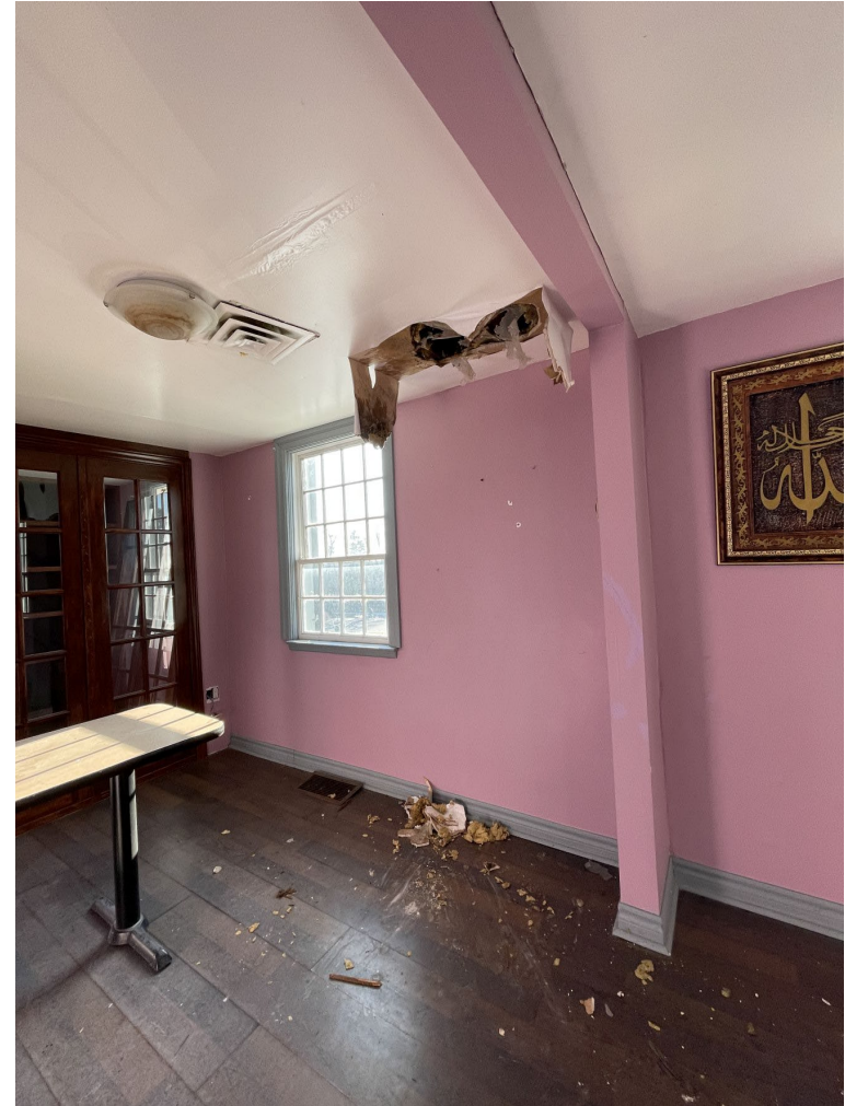
Fig. 33 Hole in the upper floor's ceiling near the building's west-facing front facade
