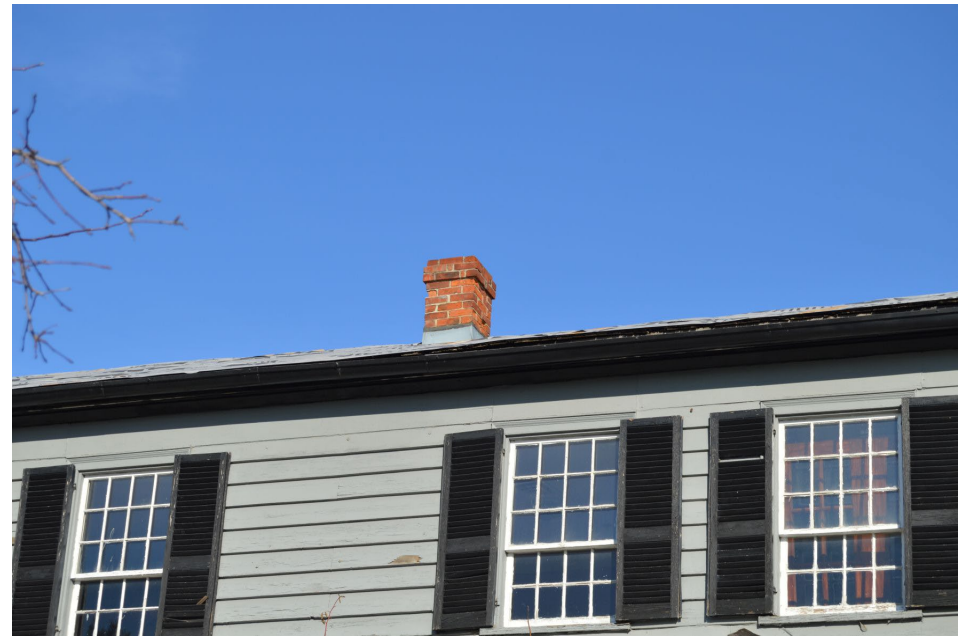
Fig. 29 Small red brick chimney on the ridge of the gable roof surmounting the house's front part
