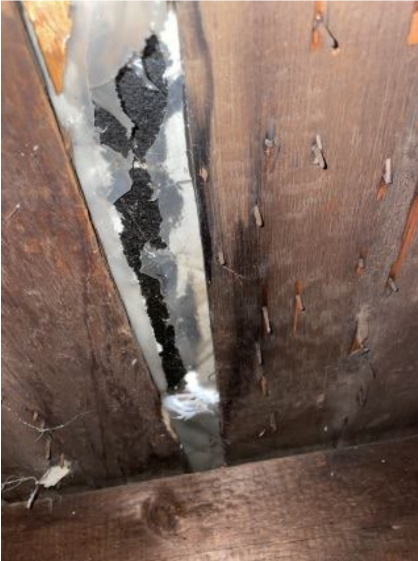
Fig. 40 Detail of the same attic's ceiling, showing a damaged asbestos sheet
