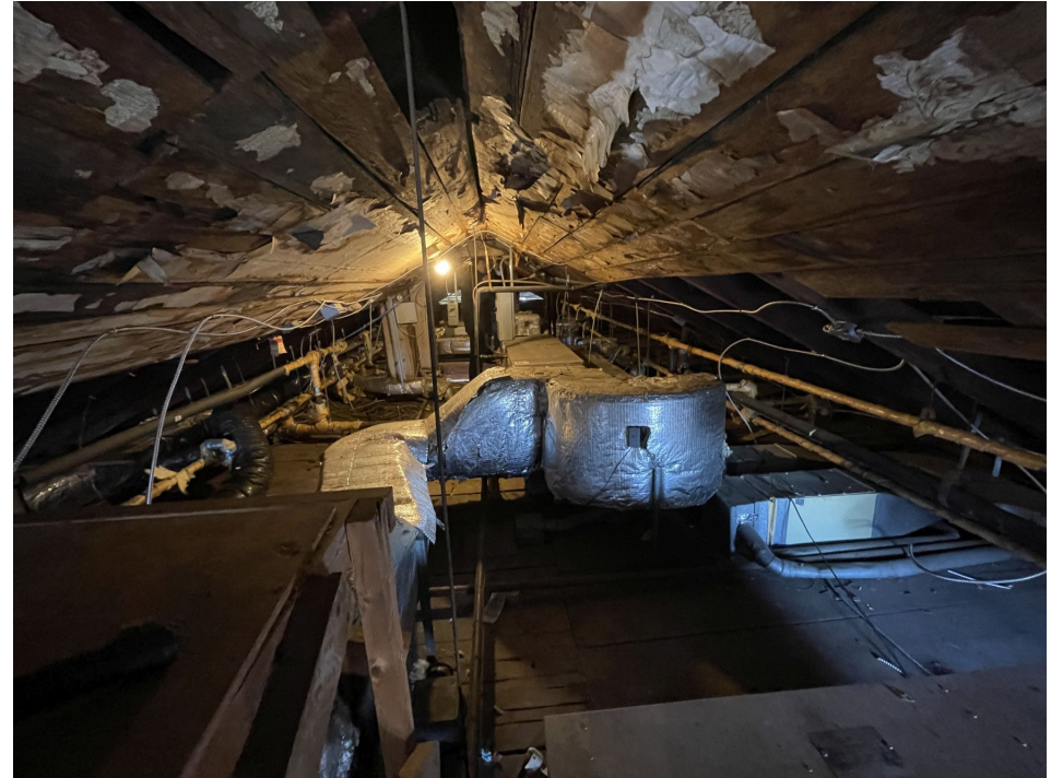
Fig. 35 View of the attic over the building's frame front part, looking south
