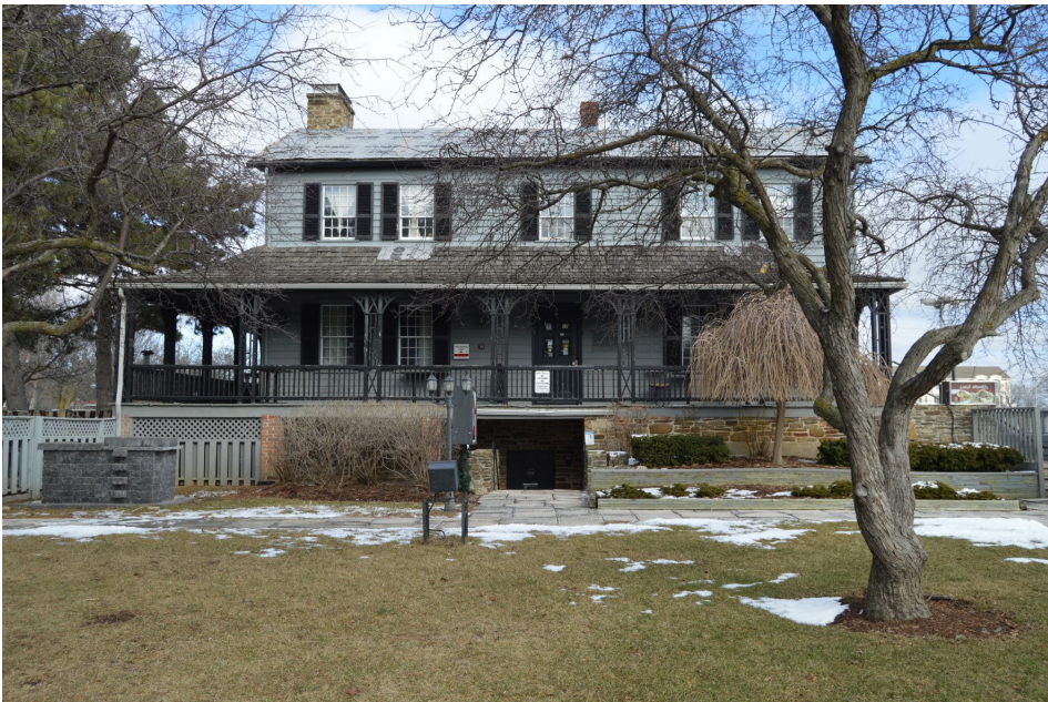
Fig. 18 Front facade (west elevation) of Cherry Hill House in 2023. Note the wood shingle cladding over the awning-form verandah roof and patches atop the wood shingle. The gable roof over the house's front part is shrouded with a tarpaulin.
