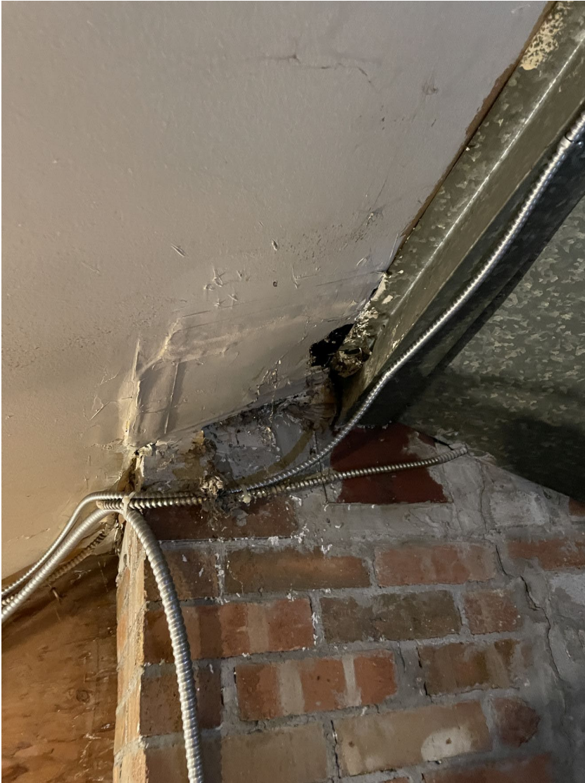
Fig. 42 View of the back wing's ceiling round its big brick chimney. Note the concrete block wall – the structure for the exterior stone veneer.
