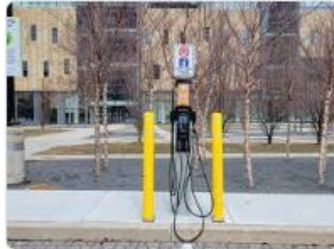
Mississauga EV Chargers
