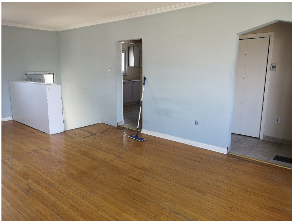
Main Floor Living/Dining Room – note evidence of renovations here – baseboards mis-match at wall openings
