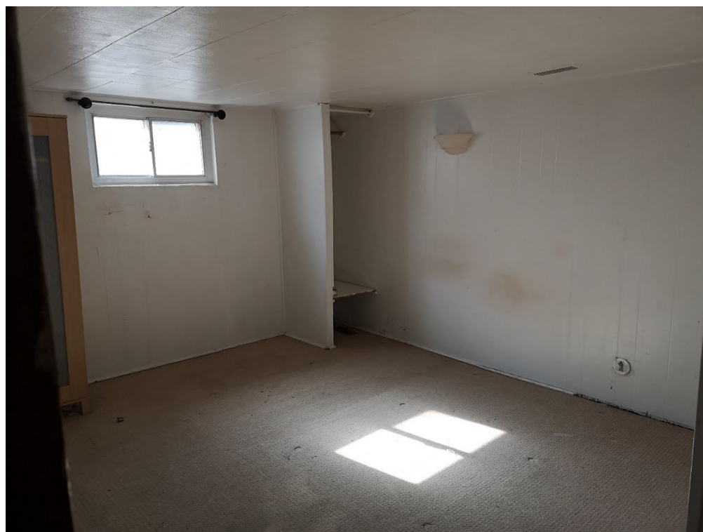
Basement Bedroom (typical) – note non-professional construction
