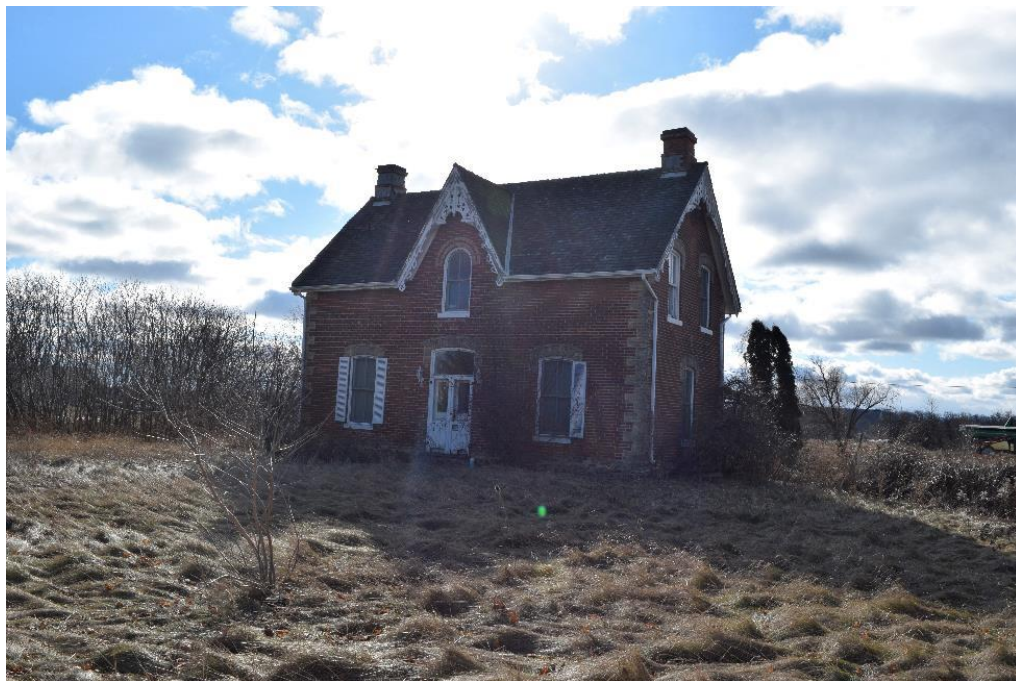
Image 9: North exposure of Britannia Farmhouse, note undersized and missing shutters.
