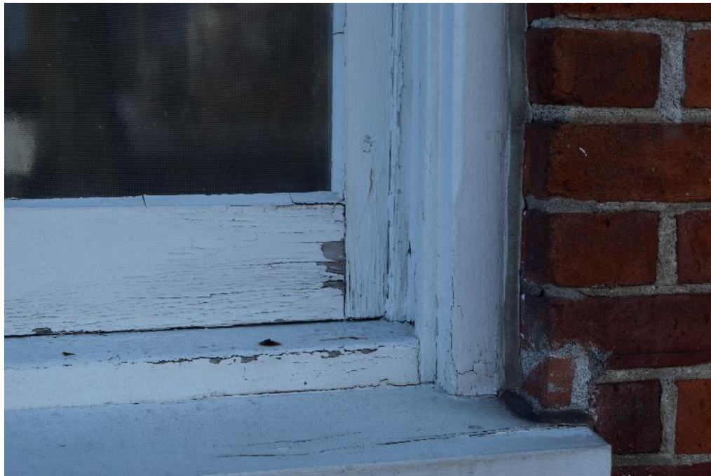
Image 6: Typical example of paint failure observed on window sash and external trim.
