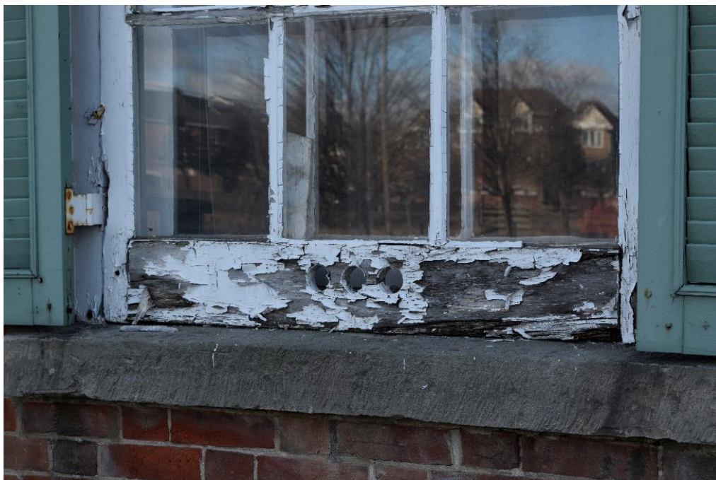
Image 22: Representative example of degradation of wooden elements, result of a lack of seasonal preventative maintenance.
