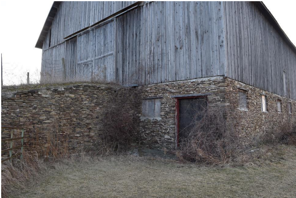
Image 25: Northwest exposure of reconstructed stone foundation under Conover Barn, note plywood covering on all windows.
