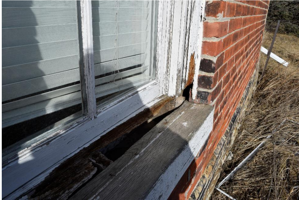
Image 14: Example of total failure of structural trim resulting in exposure of interior wall cavity.
