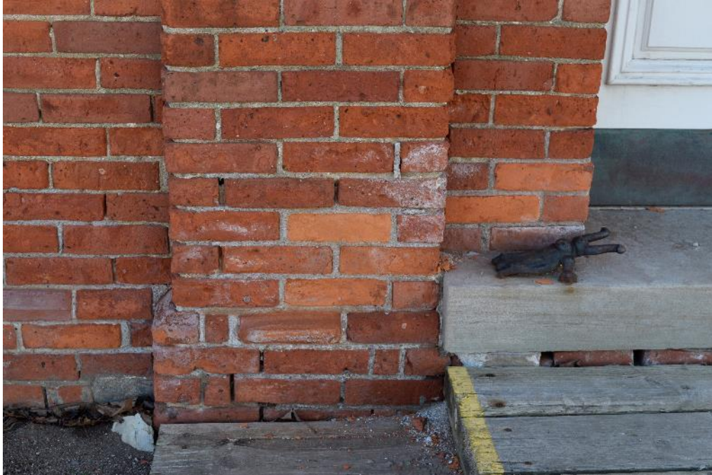
Image 5: Spalled brick and mortar damage, typical of that observed around main entrance.
