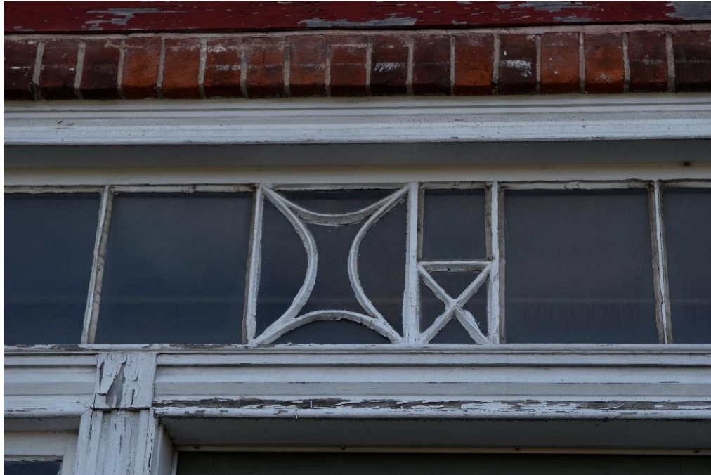
Image 21: Degradation of decorative tracery in main entrance transom.
