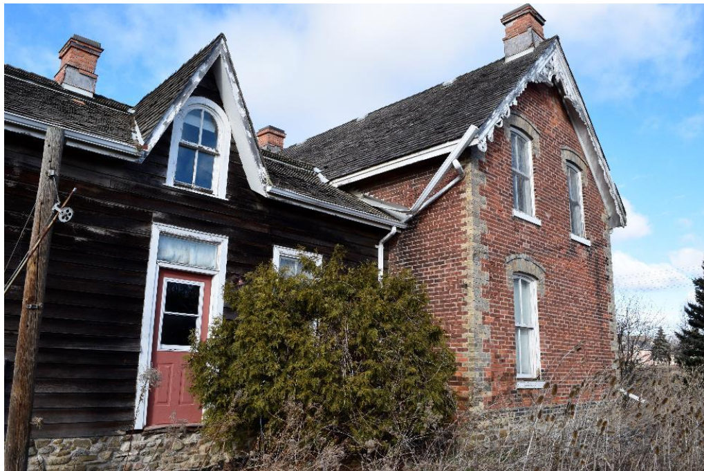
Image 11: Junction of main house and rear wing, note damage to eavestrough.
