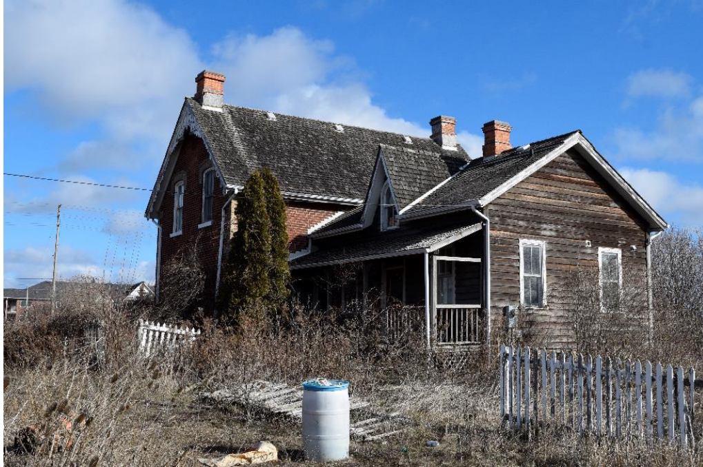
Image 12: Southwest exposure of Britannia Farmhouse, note degradation of cedar shake roof and lack of property maintenance.
