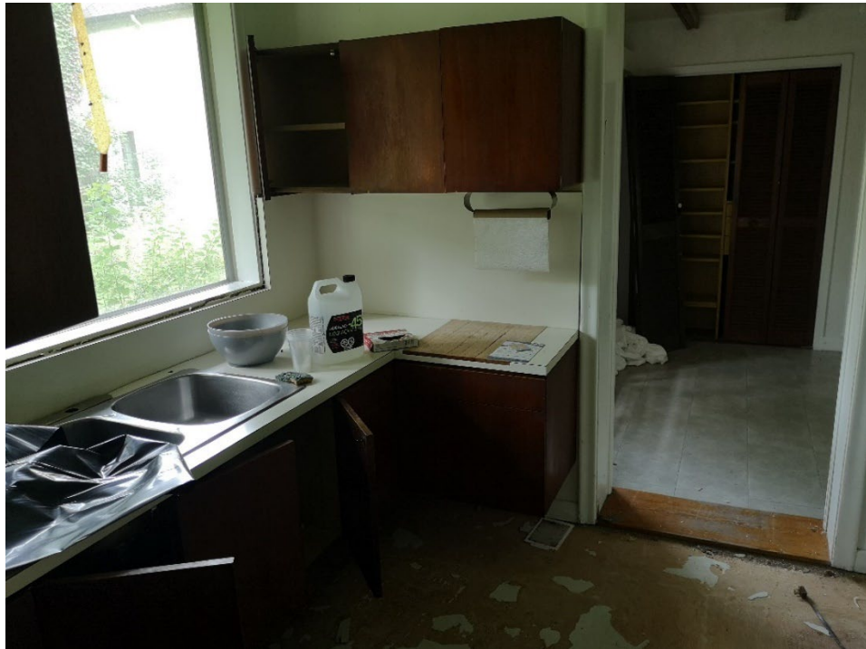
KITCHEN. NOTE FLOATING LOWER CABINETS. THE KITCHEN FLOOR HAS BEEN REMOVED FOR SOME UNKNOWN REASON.
