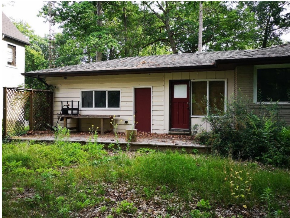
PARTIAL REAR ELEVATION. NOTE DIS-SIMILAR ALUMINUM SIDING AT CENTER BREEZEWAY
