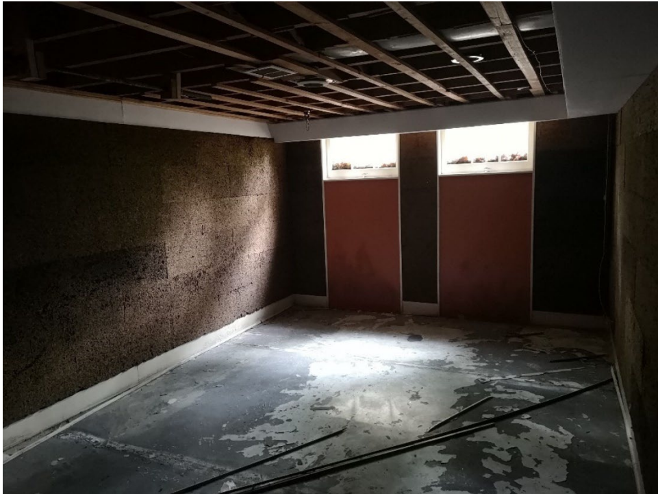
BASEMENT FAMILY ROOM. CEILING FINISHES HAVE BEEN REMOVED FOR SOME UNKNOWN REASON
