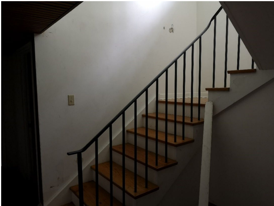
LOWER HALL AND BASEMENT STAIRS. NOTE CONTEMPORARY RAILING DETAIL, ABSENCE OF BASEMENT DOOR AT TOP OR BOTTOM OF FLIGHT
