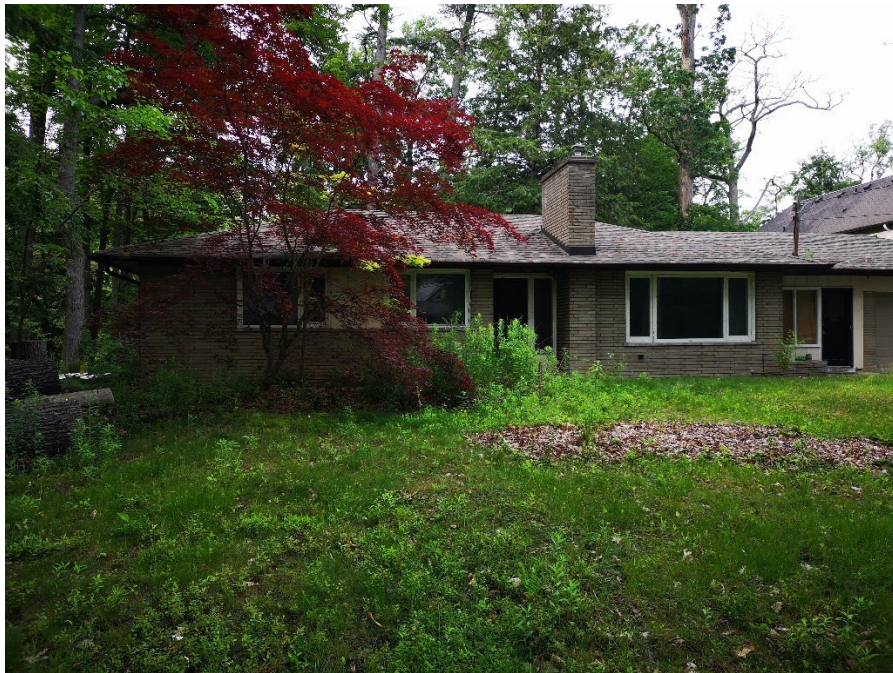
PARTIAL FRONT ELEVATION SHOWING REMNANTS OF LANDSCAPING AROUND BUILDING, GENERAL DETERIORATION
