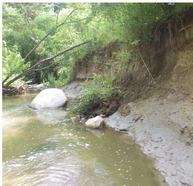
Figure 4.7. Sawmill Creek is in need for rehabilitation, as erosion impacts the channel banks and woody debris, posing significant risks to the adjacent trail, sanitary sewer infrastructure and the environment.
