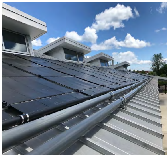
Figure 4.14. Solar panels at the Lions Club of Credit Valley Outdoor Pool exemplify the use of a renewable energy source.
