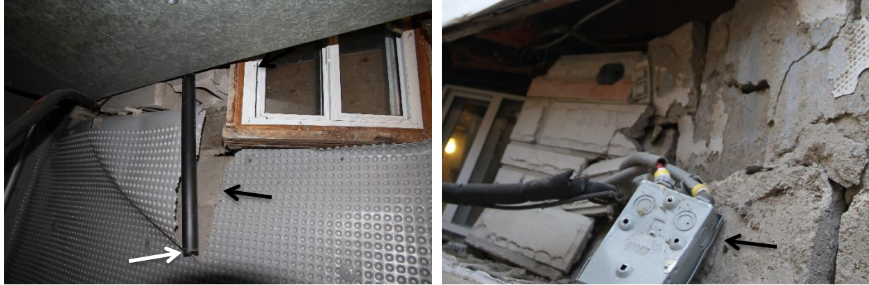
Figure 3 – Views of some of the non-structural damage observed within the affected area.
