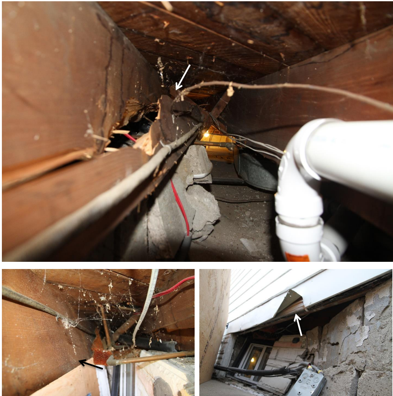
Figure 2 – Views of damaged floor joist, slightly displaced rim board, and split wood nailer on the rim board.
