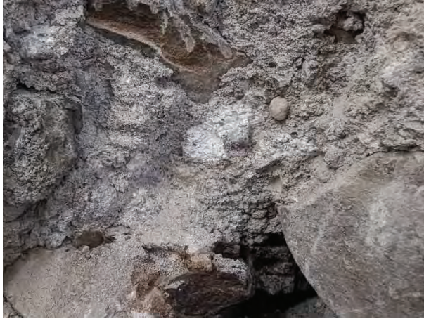
Photo #9: Typical area of concrete-masonry wall showing localized stones embedded randomly in a cementitious matrix [JCAL 2024]
