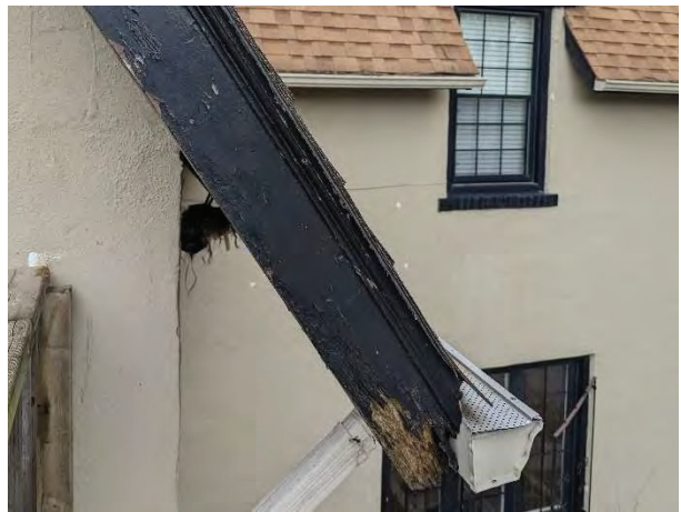
Photo #20: Rotted rafter ends [JCAL 2024]
