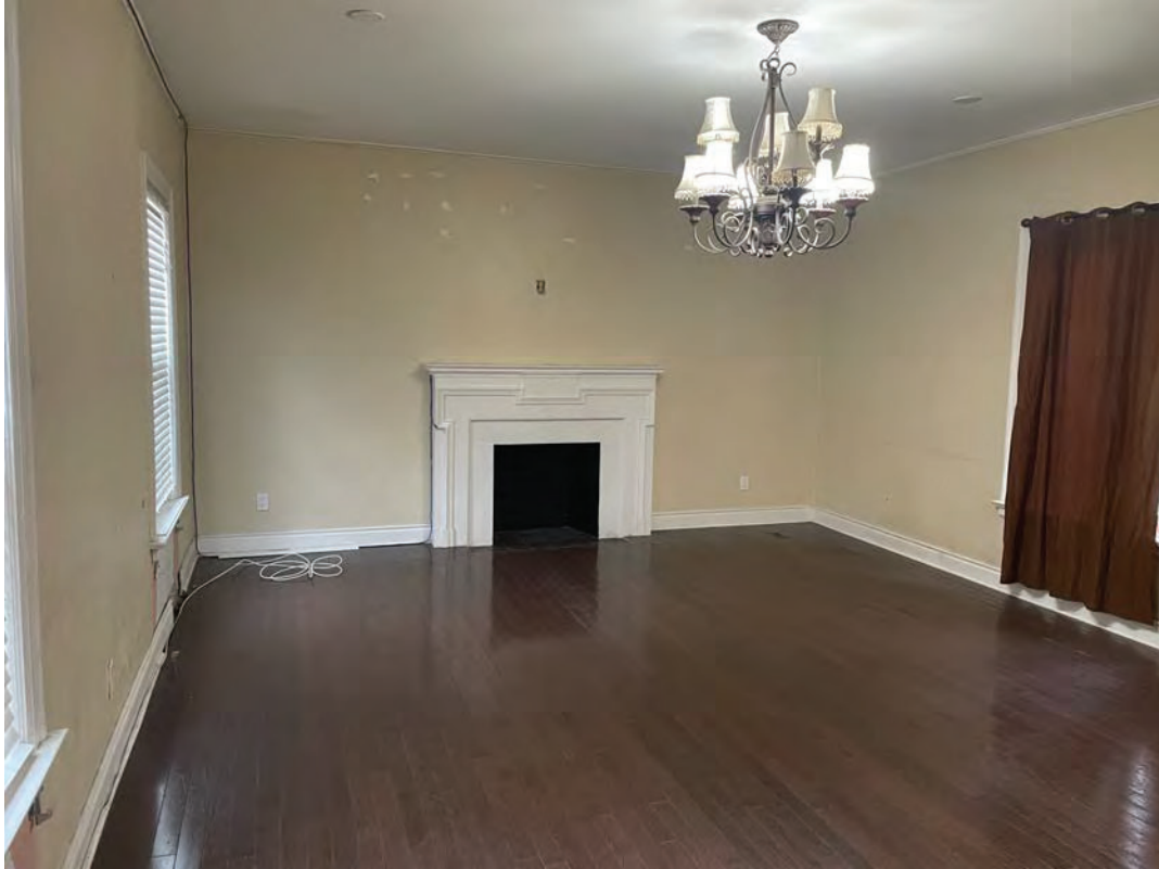
INTERIOR – 1 ST FLOOR – ADDITION TO BE REMOVED – FIREPLACE WITH STONE OR CONCRETE SURROUND
