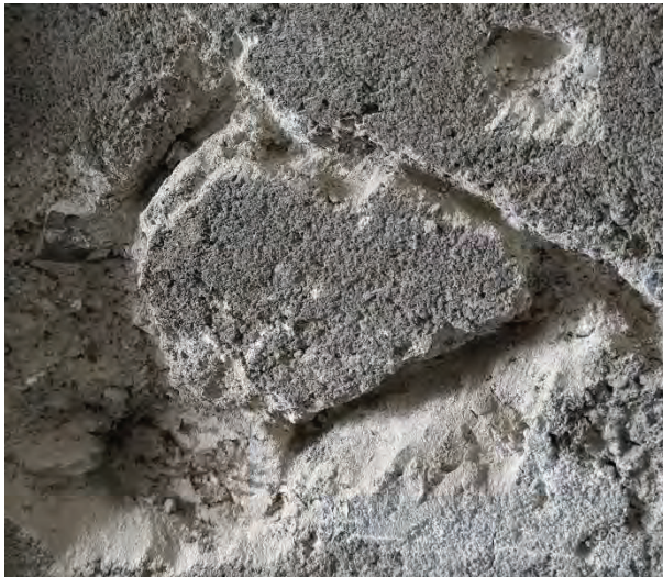
Photo #11: Easily damaged concrete-masonry wall with hand tools, typical [JCAL 2024]
