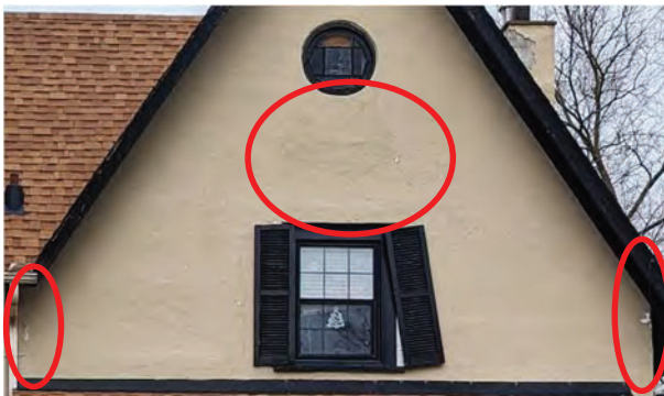
Photo #13: Previous parging repairs, and cracked/peeling parging/paint on the West Elevation [JCAL 2024]
