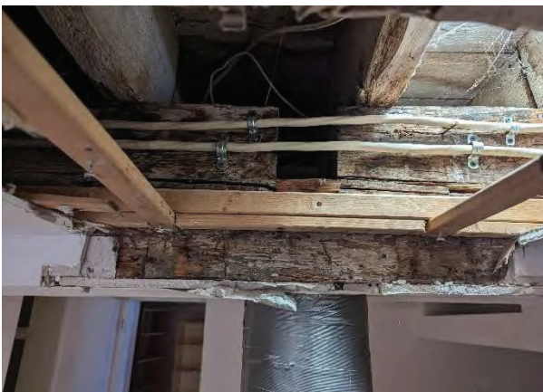
Photo #15: First-floor framing showing the wood joists supported by a notched wood beam and a circular wood column [JCAL 2024]
