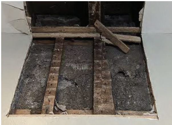
Photo #5: East exterior wall at the underside of the second floor as exposed from the interior face [JCAL 2024]
