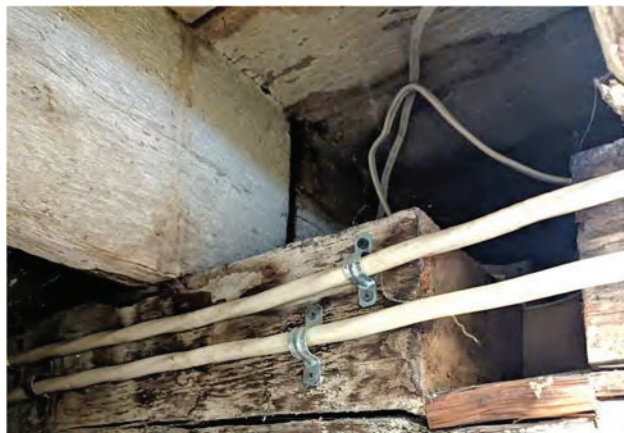
Photo #16: Butt joint at the first-floor framing joists centered above the supporting beam [JCAL 2024]
