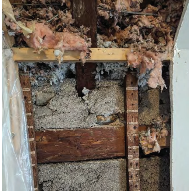
Photo #18: Exterior wall at the intersection with the roof framing showing a wood rafter extending through the wall and beyond the embedded wood top plate [JCAL 2024]
