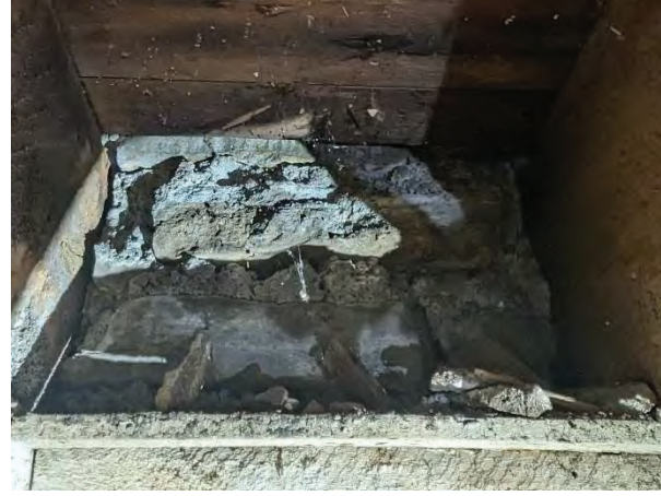
Photo #10: Stones laid in courses where the second-floor joists are embedded in the exterior wall [JCAL 2024]
