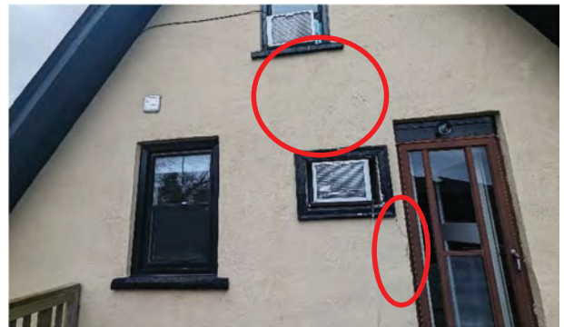
Photo #14: Cracked parging and moisture staining on the East Elevation [JCAL 2024]
