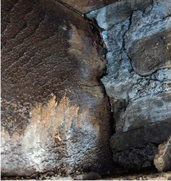
Photo #17: Rotted joist end at a second-floor joist embedded into the exterior wall [JCAL 2024]
