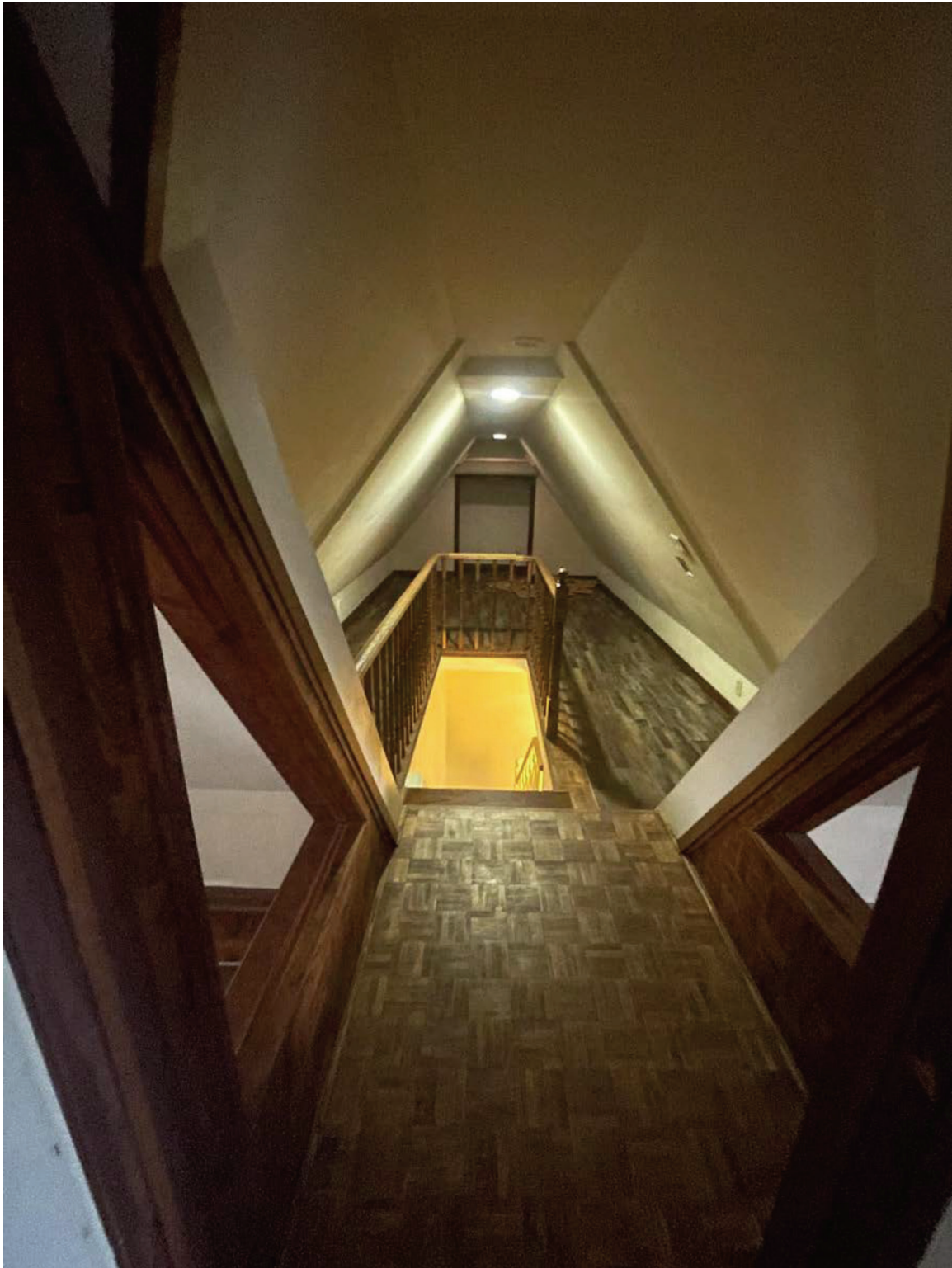
MODIFIED ROOFLINE WHERE THE 2 ND FLOOR ADDITION IS ATTACHED – ORIGINAL ROOF FRAMING PARTIALLY PRESERVED BENEATH THE LATER ADDITION
