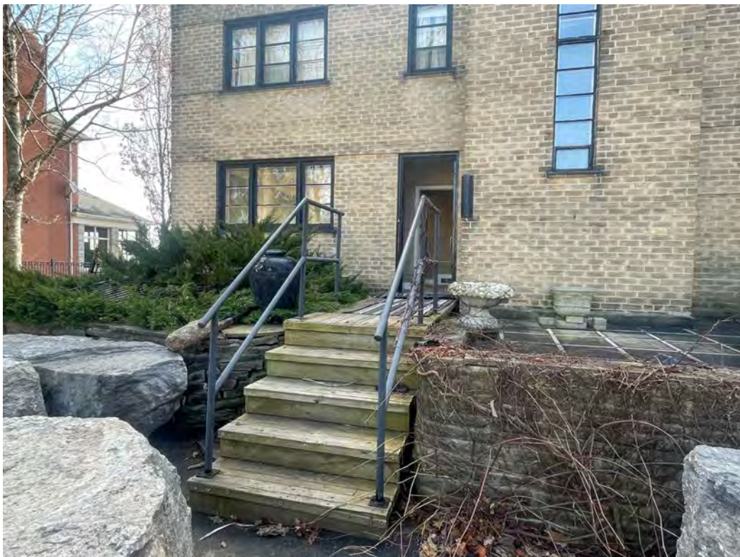
WOOD STEPS & METAL HAND RAILS AT THE FRONT ENTRANCE (original stone steps maybe below?)
