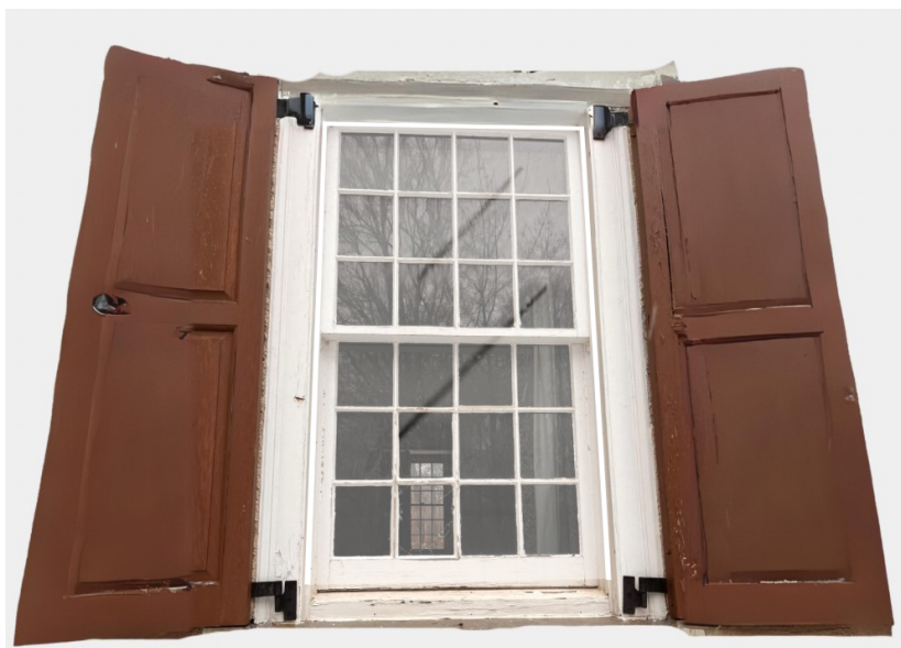
Mock-up of a typical window with a Lexan panel and white trim across the top and down the sides.
