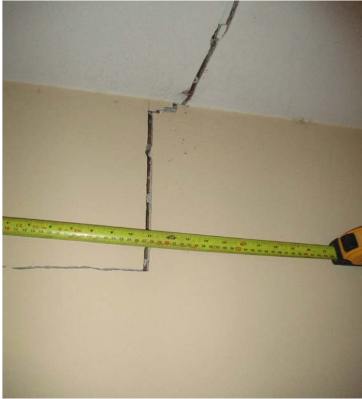
Pic. 3 Second floor interior wall finish cracks over the garage
