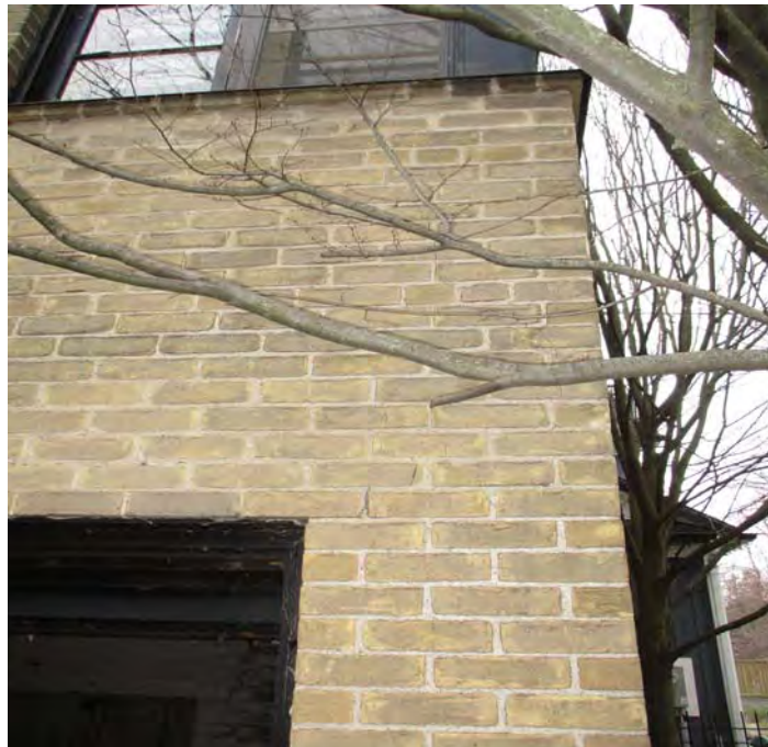
Pic. 4 Second floor brick masonry cracks over garage
