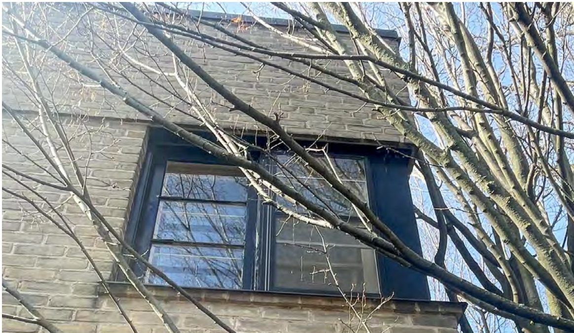
EAST ELEVATION (DETAIL) - showing the glazing pattern, wood frame and brick rebate of the corner window – showing the projecting brick sill below the window and the raised brick band level with the window top
