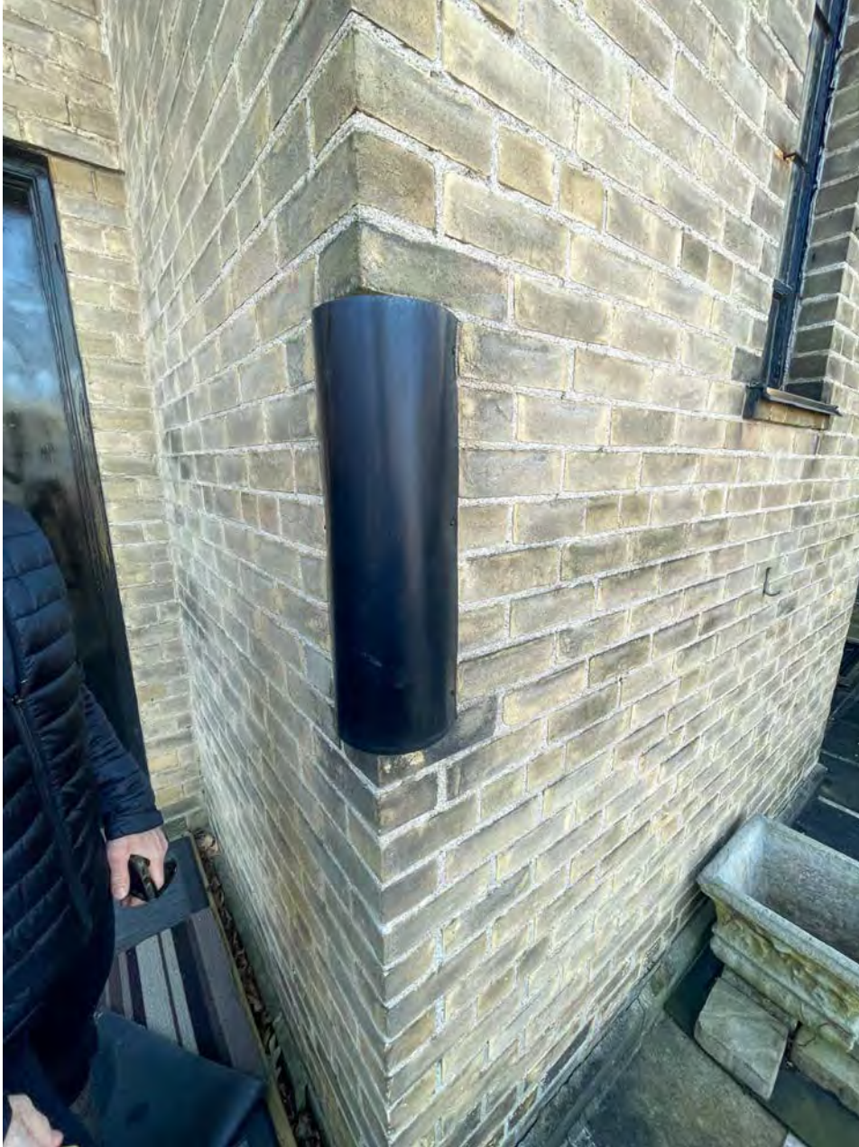
EXTERIOR LIGHT FIXTURE? (appears to be an original feature set into the brick corner that may be intact beneath the protective covering)
