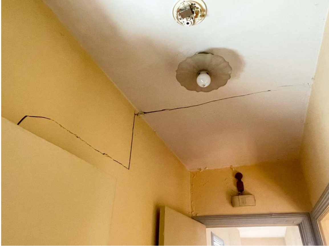
INTERIOR – GARAGE LINK – 2 ND FLOOR – large shear crack through the plaster
