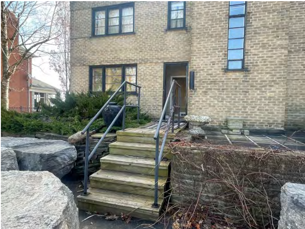
WOOD STEPS & METAL HAND RAILS AT THE FRONT ENTRANCE (original stone steps maybe below?)
