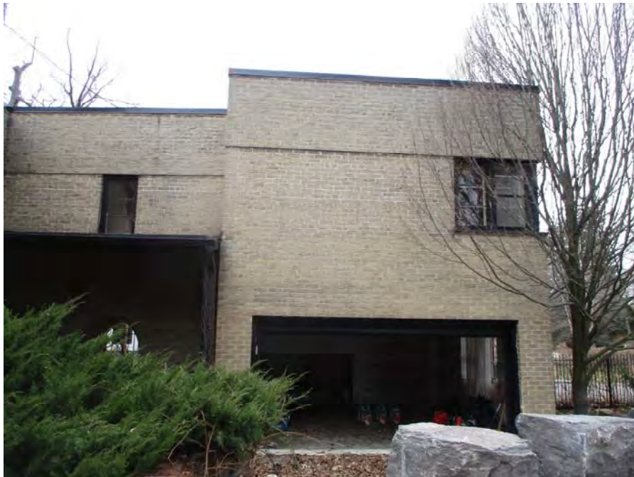
Pic. 2 60 Cumberland Dr. – Garage Elevation – slopes noticeably right (north)
