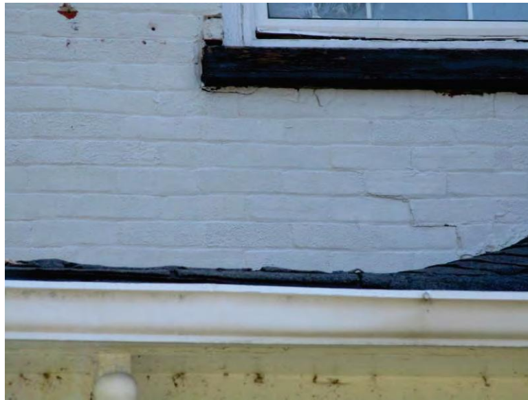
Figure 7: Step cracking below second storey window
