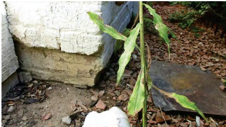
Figure 4: Deteriorated coatings near grade
