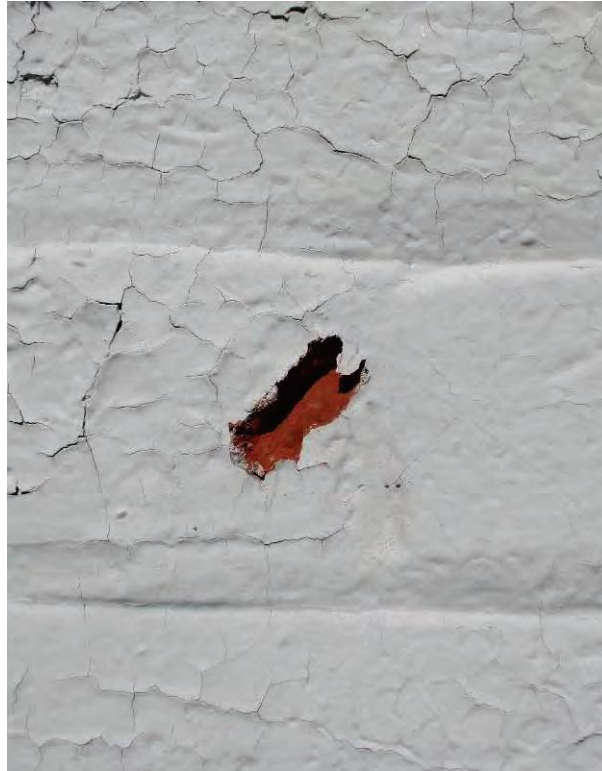
Figure 3: Soft brick exposed below coatings
