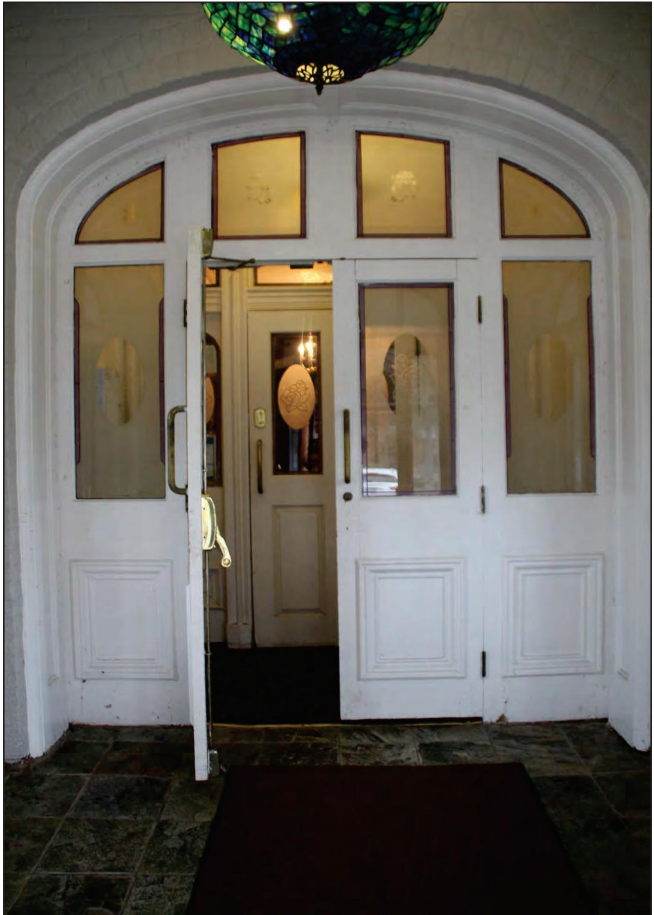
Figure 51 doors, top lights and sidelights (replacement glass & hardware) to umbrage from exterior
