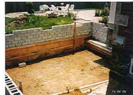
In this photo we see the foundations being laid for the family room/sunroom that was added to the building by the current owner Latiq Qureshi.
