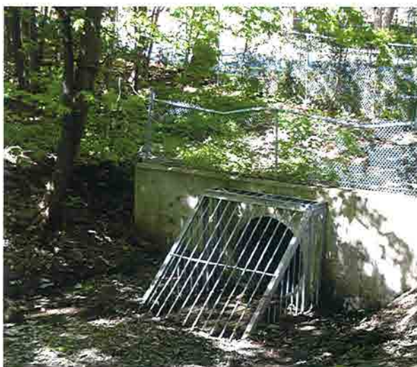
17. Storm drain as it passes underneath King Forest Drive on the east end of the property.
