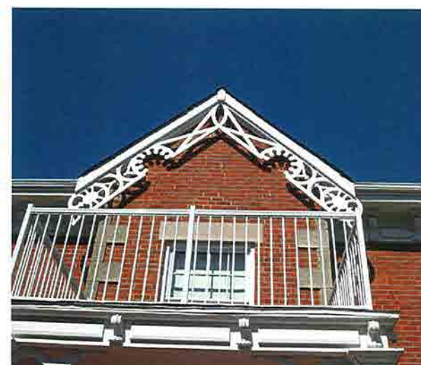
3. Vergeboarding detail on gabled front entrance: The porch and railings are not original.
