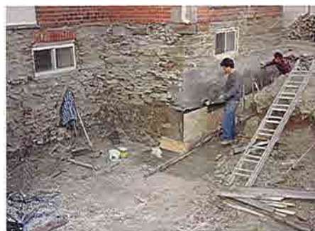
The current owner made extensive repairs and additions to the foundations of the main house such as the addition of footings and a weeping tile.
