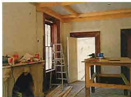
Extensive restoration work was done by the owner, Latiq Qureshi, on the interior of the building. In the photograph above we see the dining room in the process of being restored.
