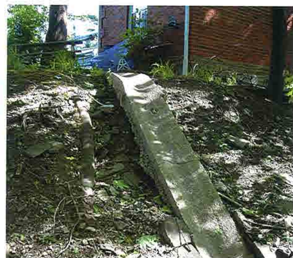
22. Concrete channel to carry runoff down to the creek. Located behind the outbuilding
