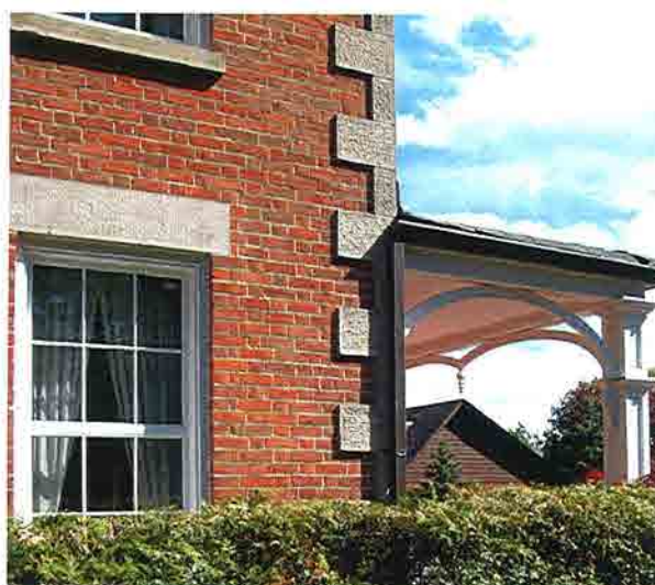
24. Stone quoins on the corners of the house. The windows have stone lintels and sills.
