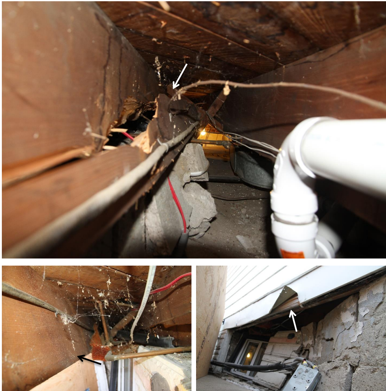
Figure 2 – Views of damaged floor joist, slightly displaced rim board, and split wood nailer on the rim board.
