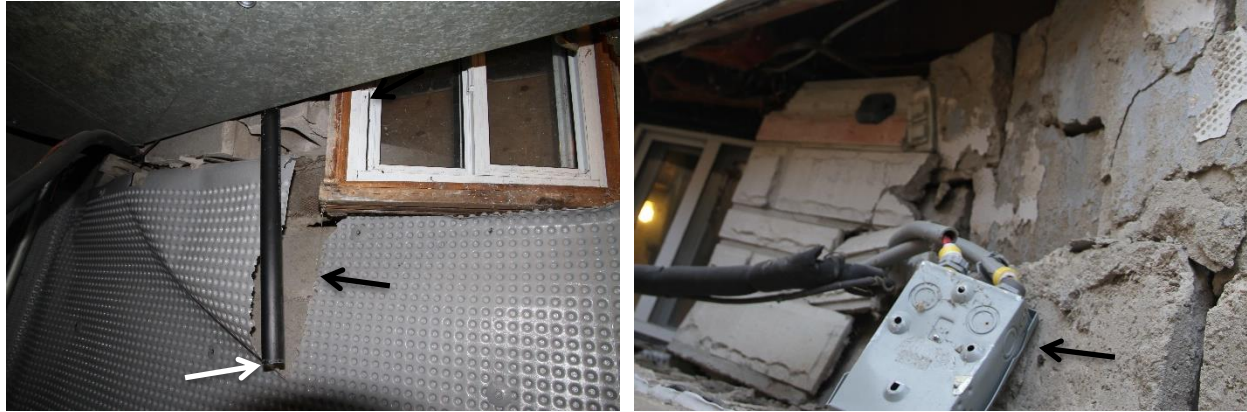
Figure 3 – Views of some of the non-structural damage observed within the affected area.
