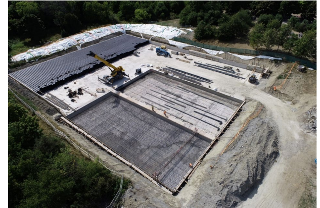
Underground Storage Facility
