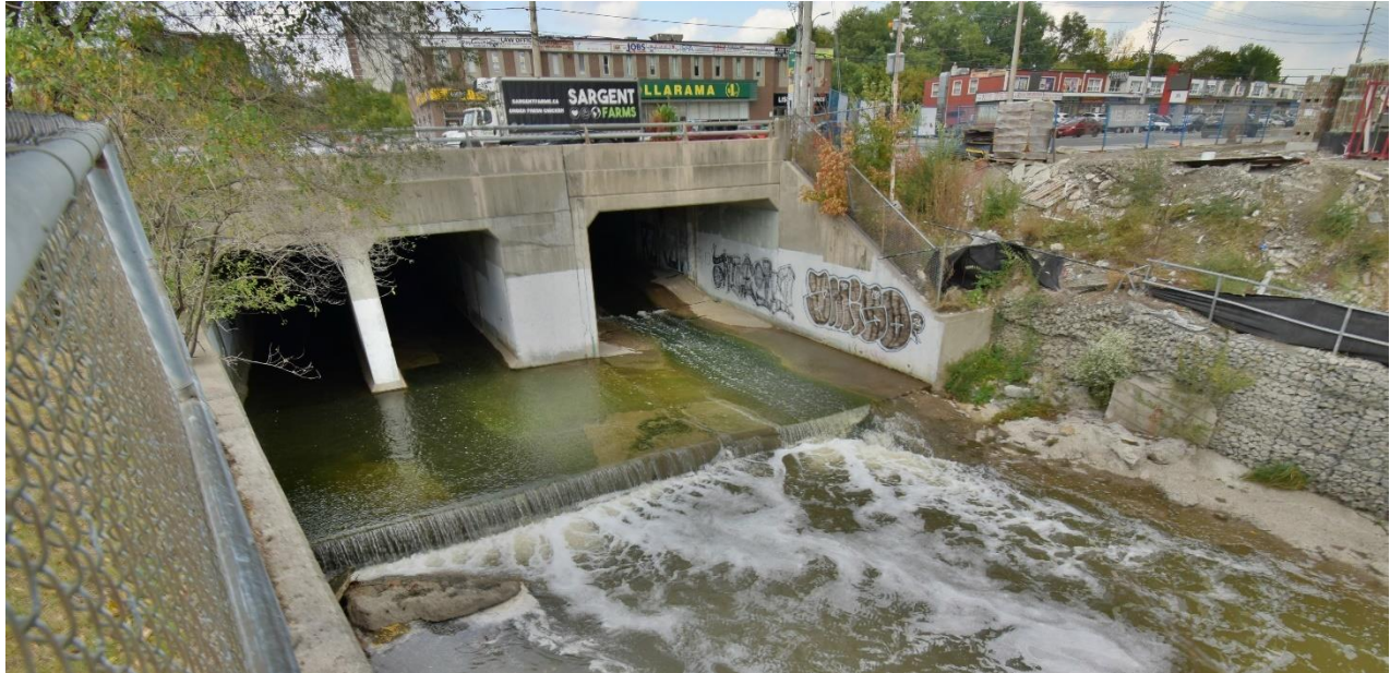
Image 1: Cooksville Creek and surrounding built and natural areas are experiencing increasing pressures due to increasing storm intensity and frequency, urban development and aging infrastructure (Credit: CVC)
