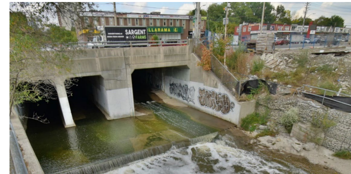
Aging infrastructure and increased stormwater runoff
