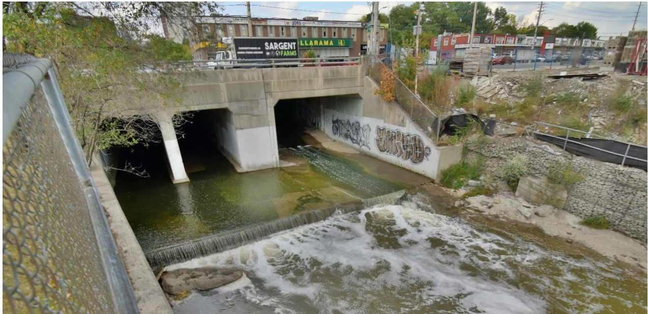
Image 1: Cooksville Creek and surrounding built and natural areas are experiencing increasing pressures due to increasing storm intensity and frequency, urban development and aging infrastructure (Credit: CVC)
