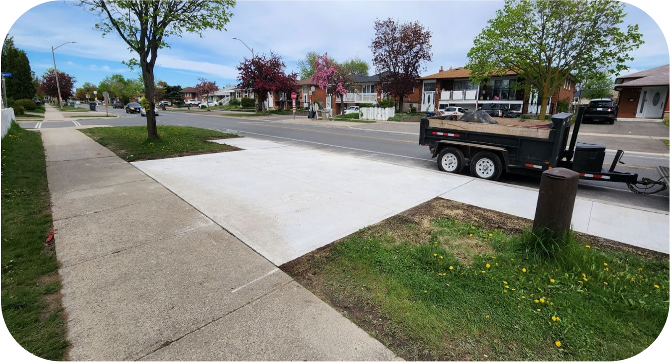
Figure 1: New customer landing pad and transit shelter pad at bus stop#2362 Morning Star Dr. at Netherwood Rd.
