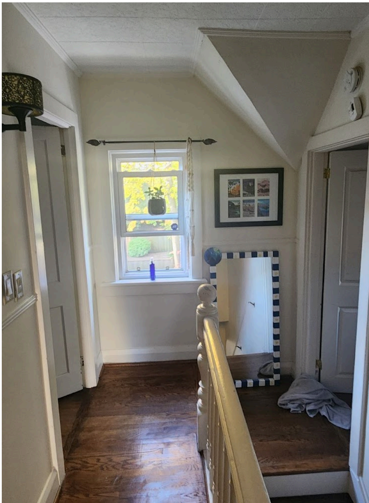
Figure 8: View of hallway at second floor showing rear window. Window opening to be extended to floor to accommodate access to new primary bedroom. (Photo by owner, October 2024)
