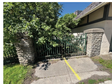
Stone piers to the south of the existing detached garage. Both the garage and the stone piers are recommended to be adapted for reuse while maintaining their relationship to 90 High Street East (ERA, 2024).
