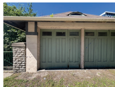
East elevation of detached garage, which is of architectural and contextual interest (ERA, 2024).
