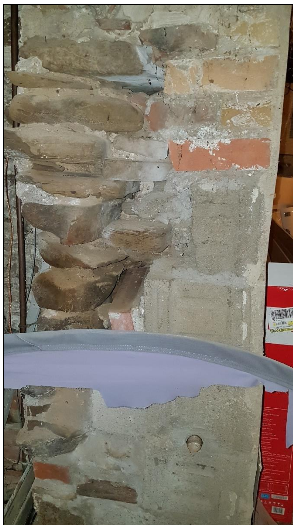
Figure 71: Portion of the foundation wall where the original stone foundation meets the concrete block foundation of the rear addition (note that portions have been repaired with brick)
