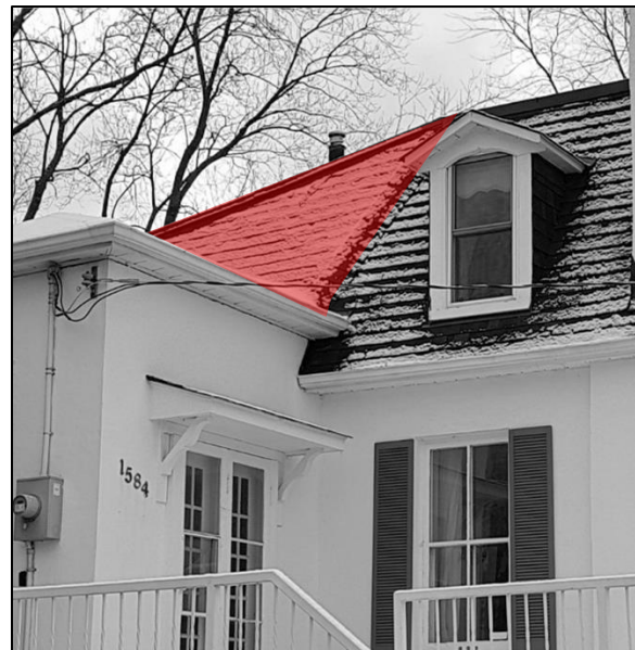
Figure 87: Photo of the extension of the mansard roof (the extension is shown in red)
