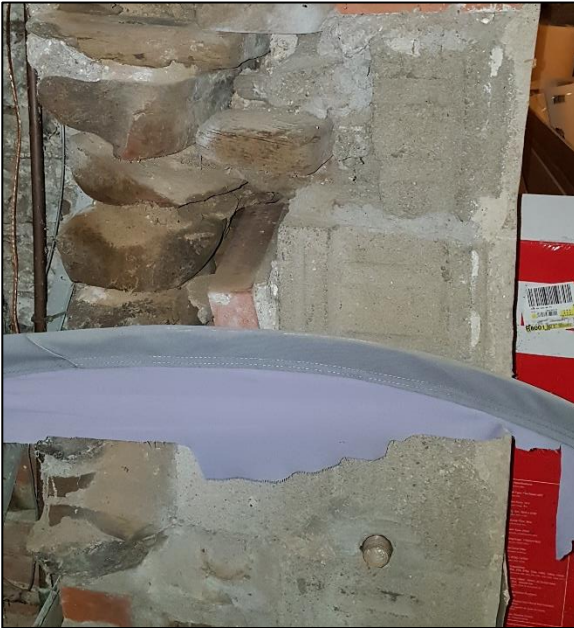
Figure 84: Photo of the stone foundation of the original building where it meets the concrete block foundation of the rear addition
