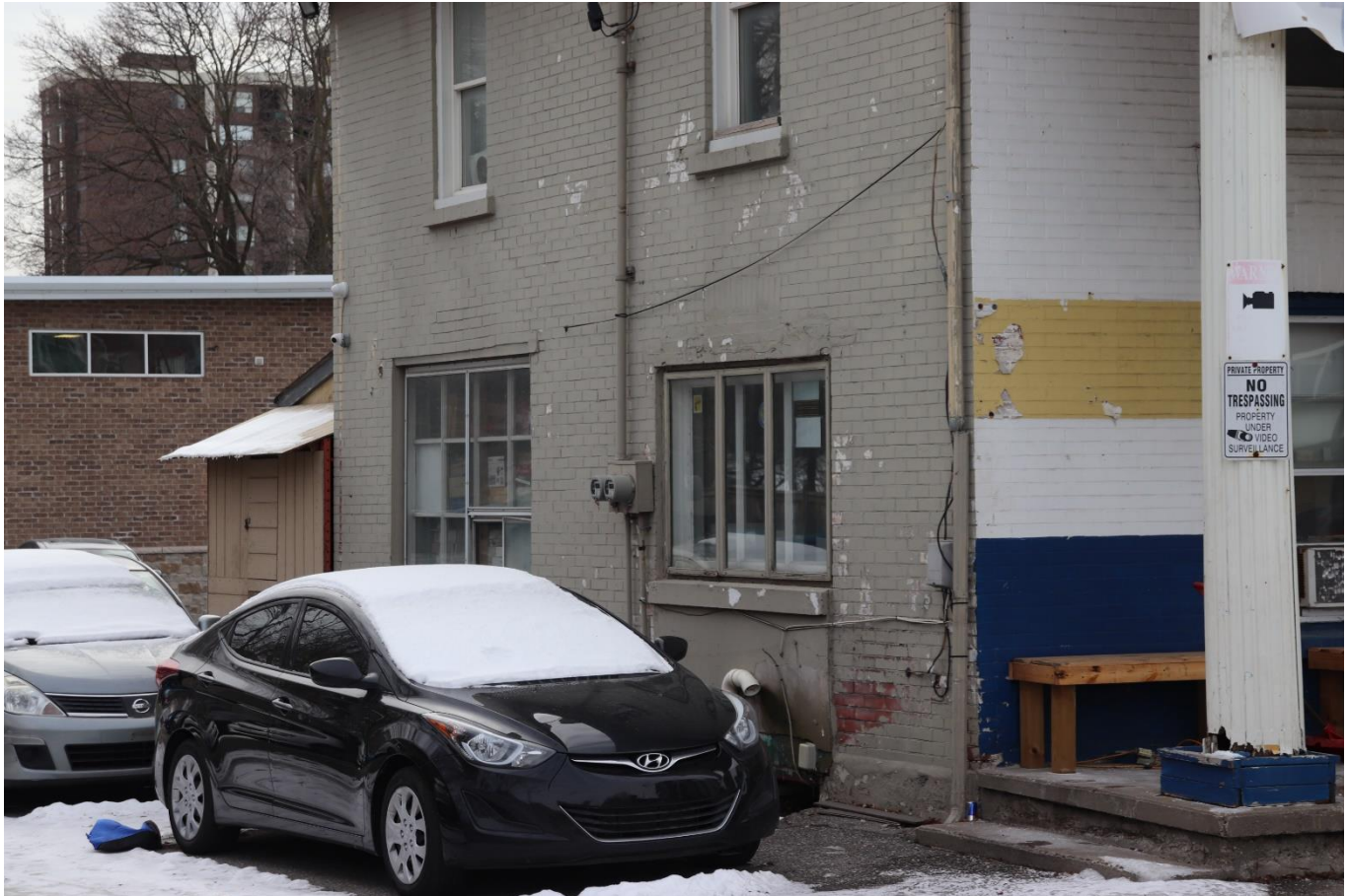
Photograph 11: View of the east elevation illustrating the aluminum three paned sliding window and the twelve-paned aluminum window, looking south (AECOM 2021)
