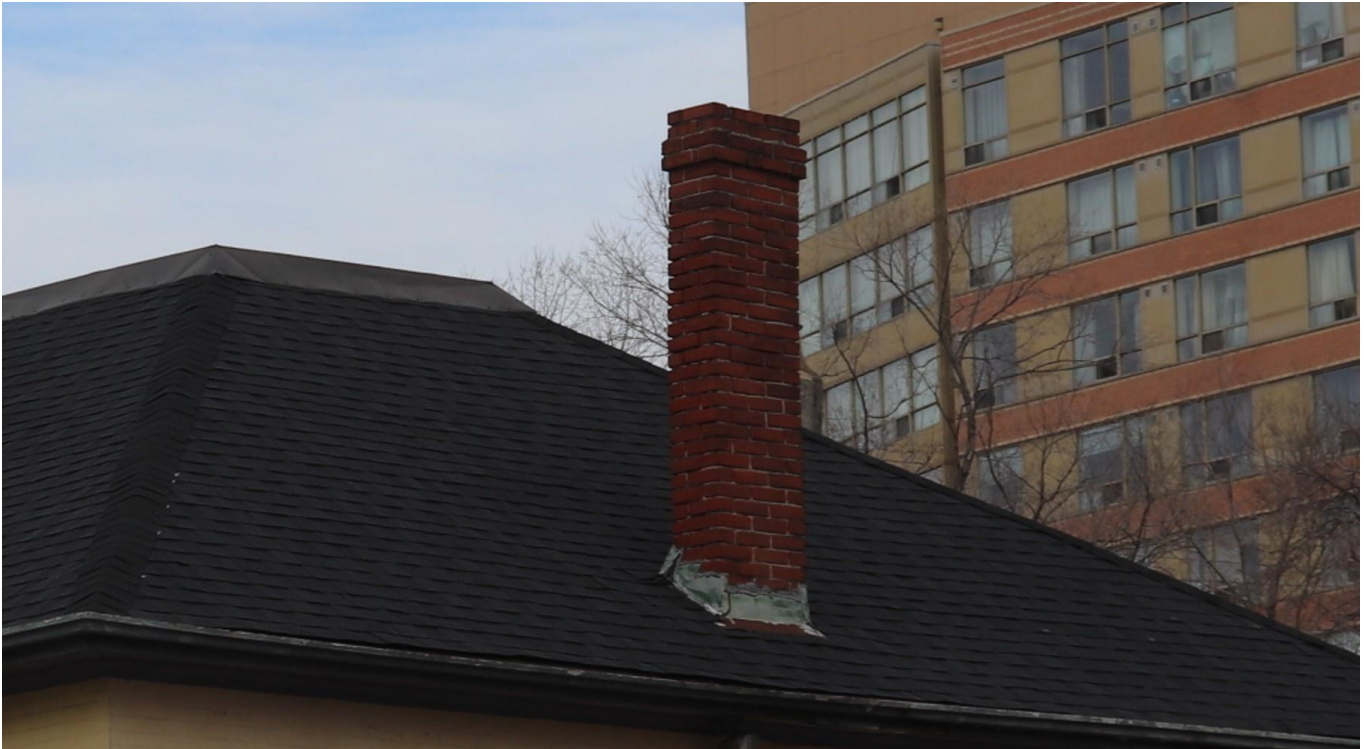
Photograph 9: View of the south elevation, illustrating the redbrick chimney, looking northeast (AECOM 2021)
