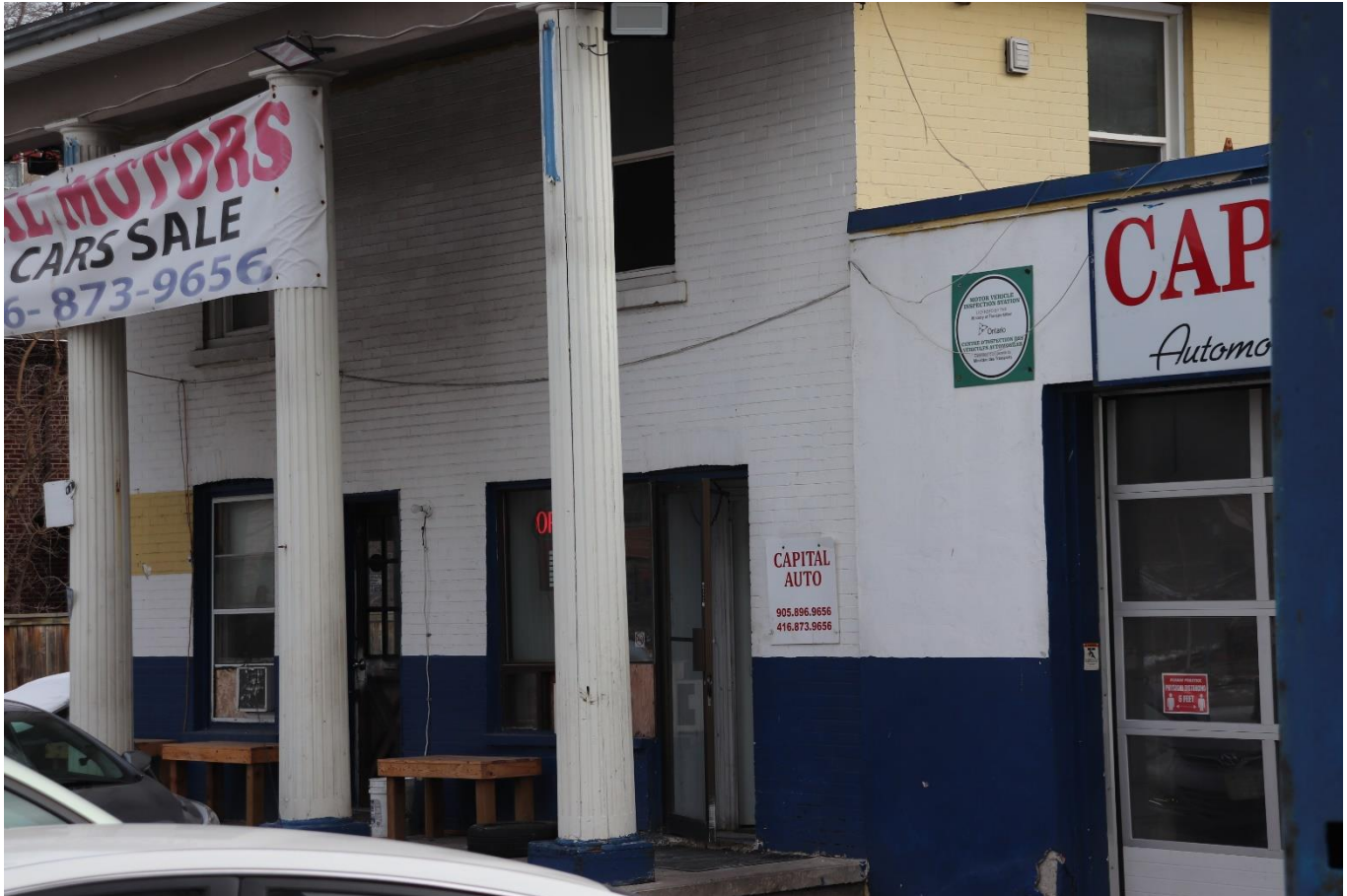
Photograph 3: View of the north elevation, illustrating the central entrance flanked by windows on either side of the doorway and the off-centre entrance, looking southeast (AECOM 2021)
