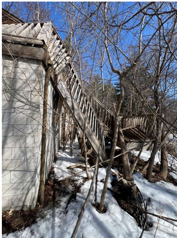
REAR DECK COLLAPSING
