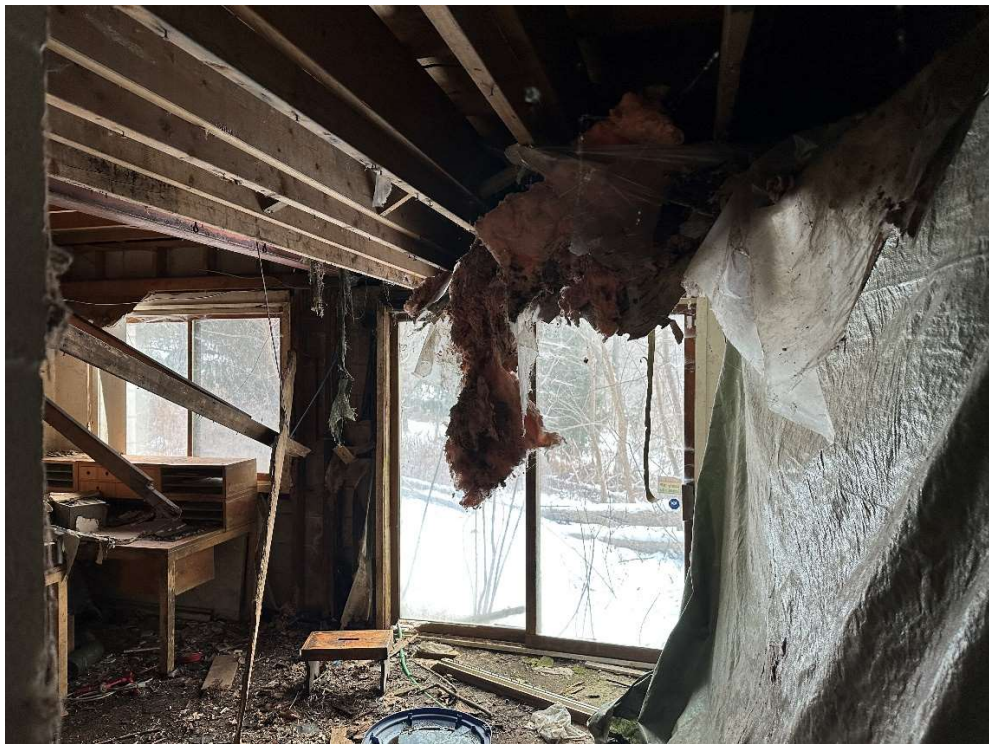
GENERAL DETERIORATION, WATER LEAKAGE
