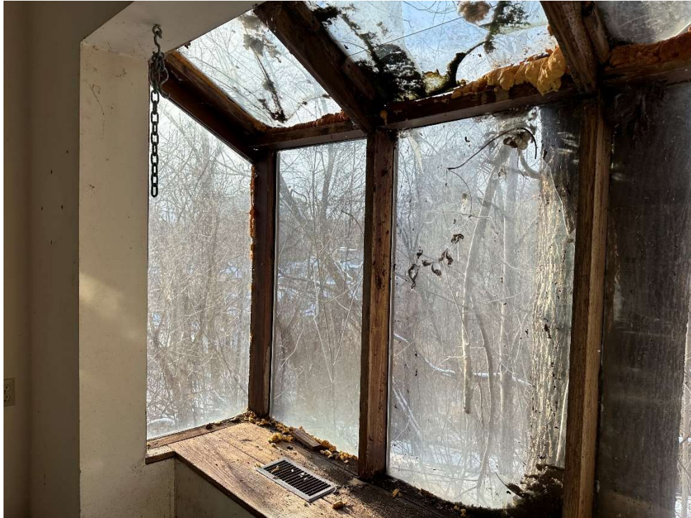
INTERIOR WINDOW DETERIORATION
