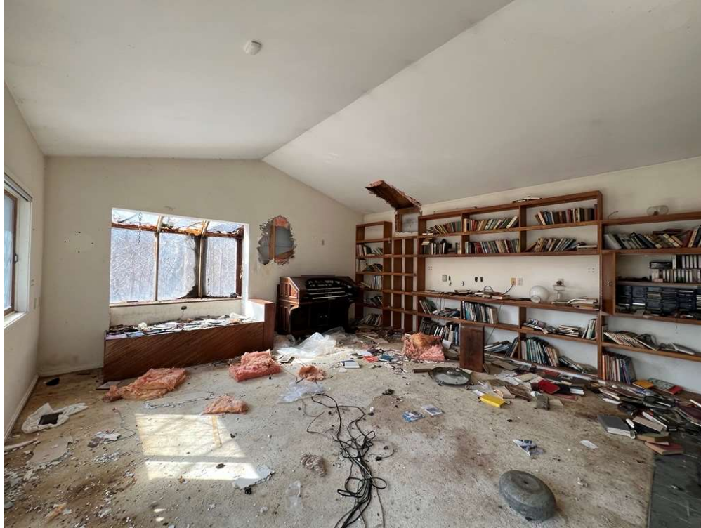
LIVING ROOM DEBRIS, VANDALISM
