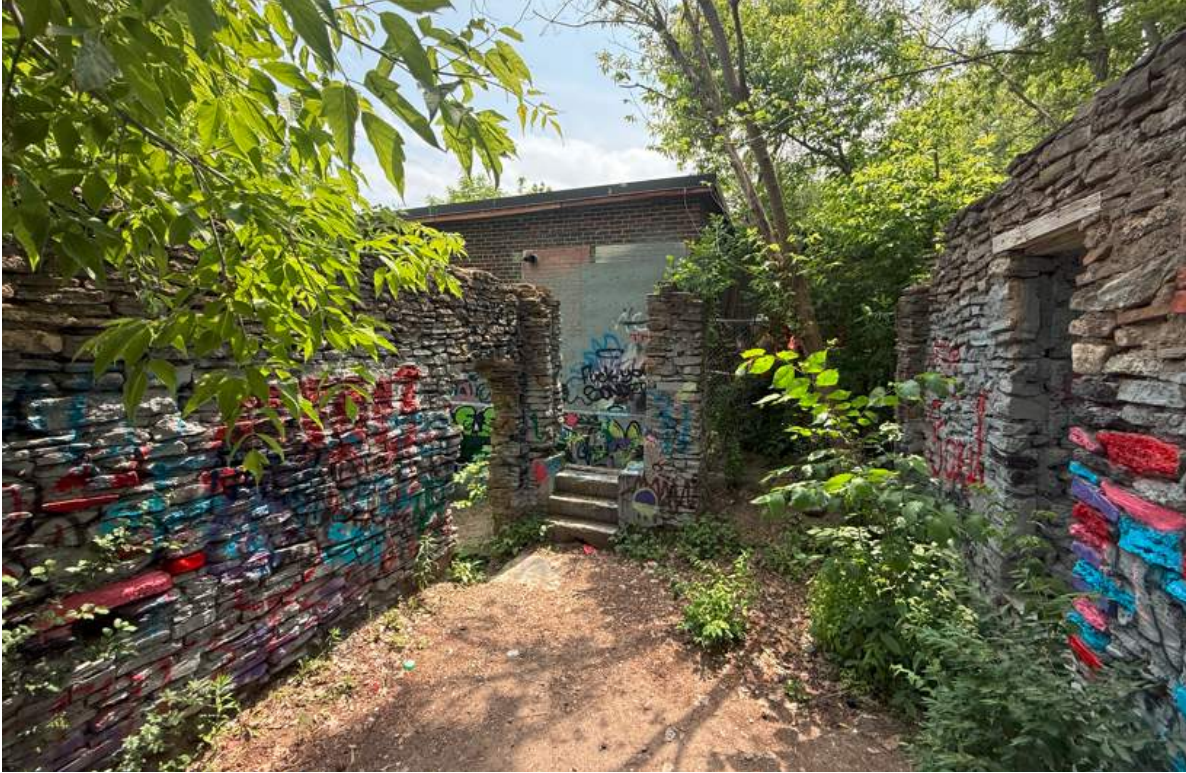
View from inside the mill toward the pump building, showing steps at the threshold, application of graffiti, and overall deteriorated conditions of the masonry walls
