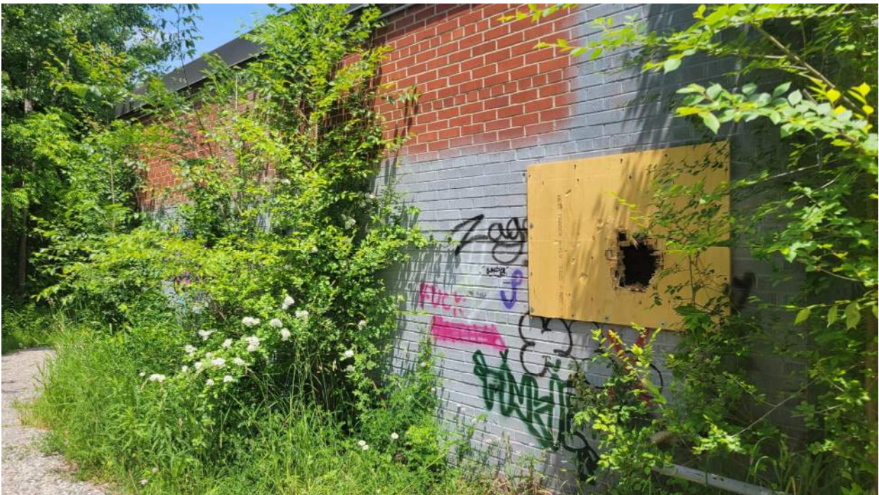
West exterior wall of pumping station building with plywood hoarding at an opening in the wall
