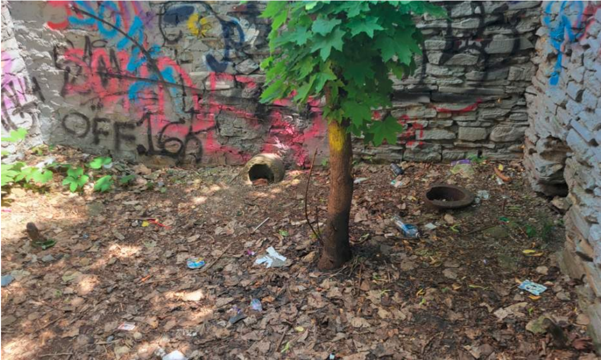
Remains of a concrete pipe through the wall
