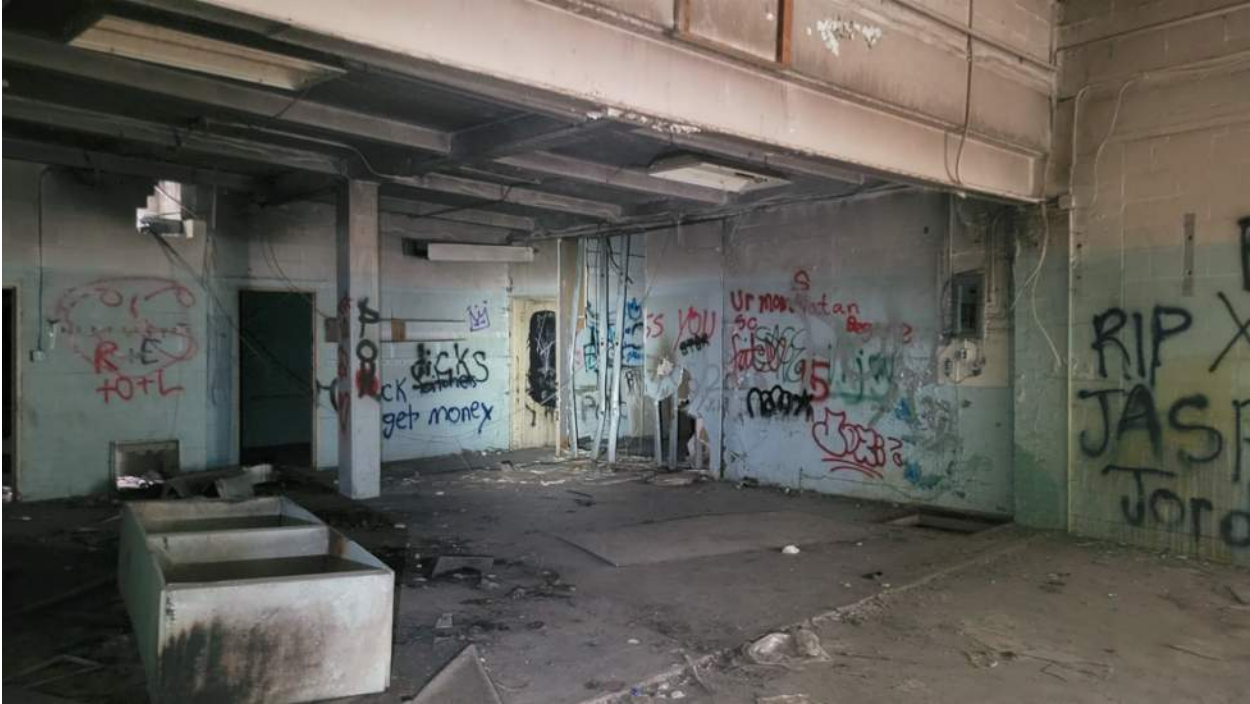
Image showing the dilapidated condition of the interior finishes
