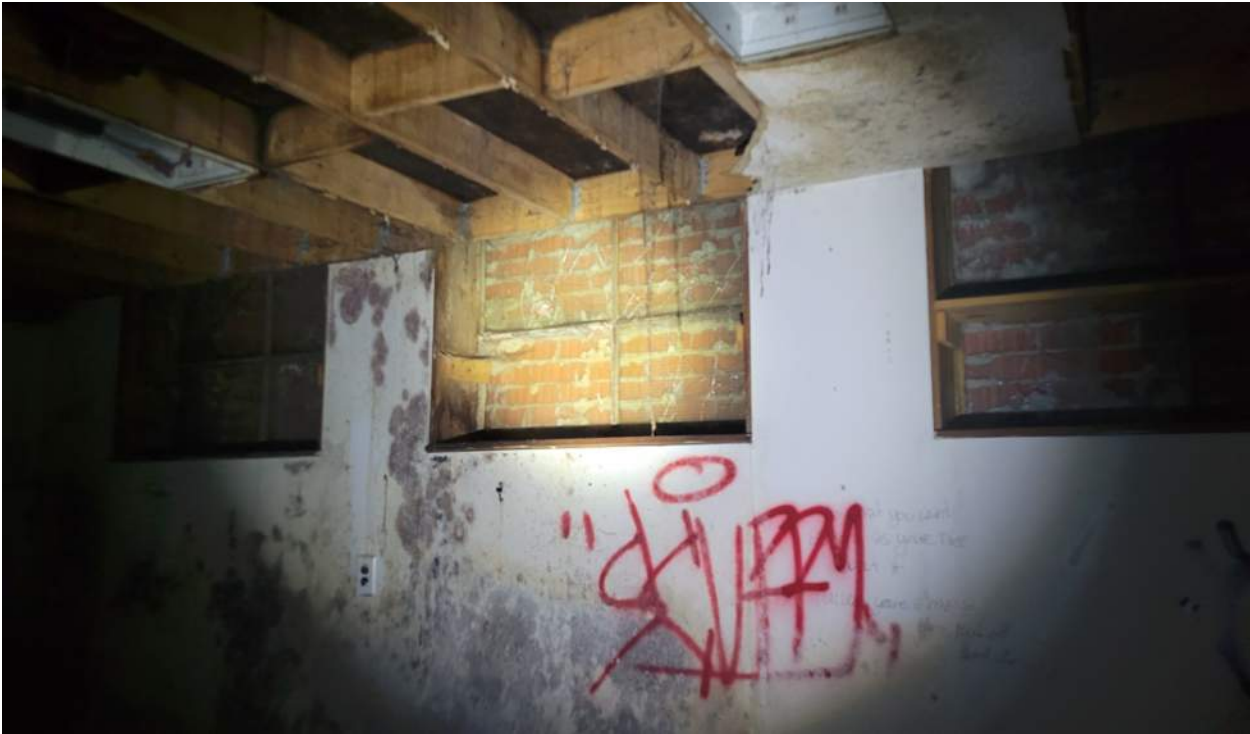
Interior view of pump house building, with mold on the walls and window openings infilled with brick
