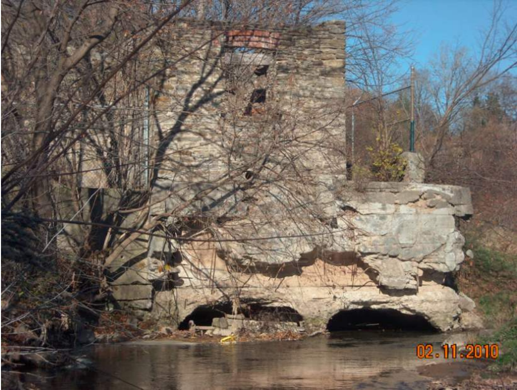
The structure of mill at the river discharge; the concrete overlay including remnants of concrete buttresses on the face of the pier may have been original (image source: City of Mississauga)
