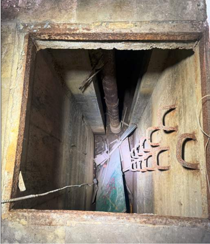
Ladder rungs into one of the below-grade pump wells.
