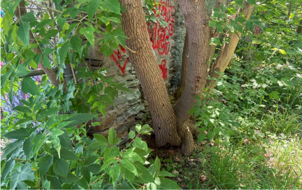
Rubble wall of the mill structure, with trees growing close to and undermining the existing wall
