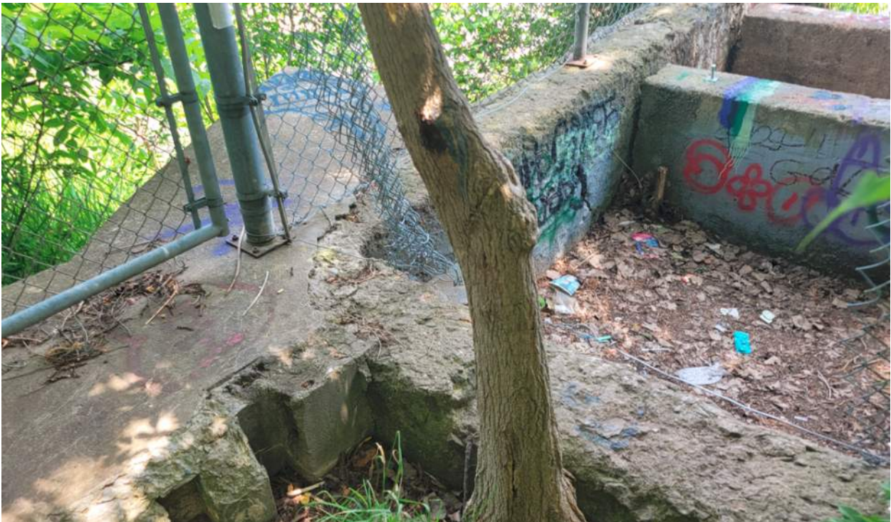
Concrete foundations belonging to a later structure attached to the original mill foundations at the corner
