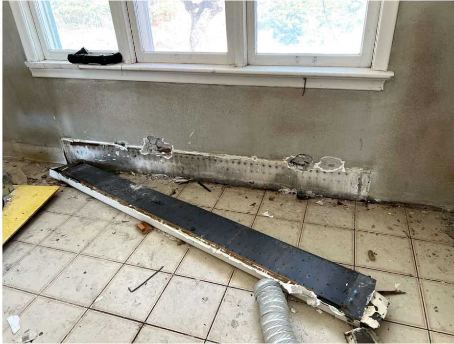
NOTE MOULD ON WALLS, VANDALISM
