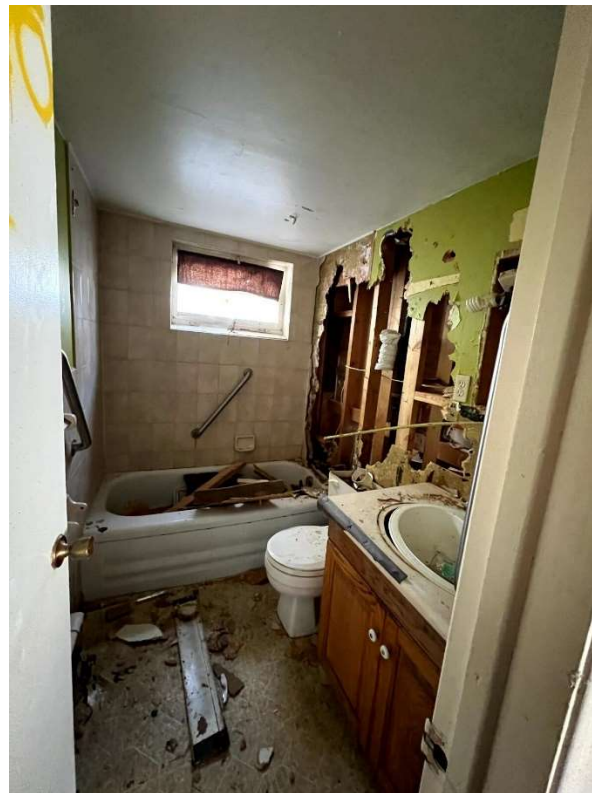
INTERIOR VANDALIZED AND ROBBED OF COPPER
