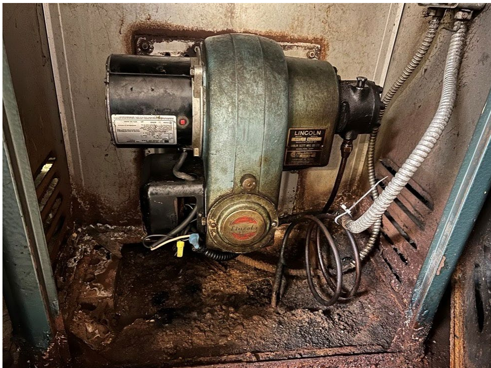
ANTIQUATED OIL BURNING FURNACE
