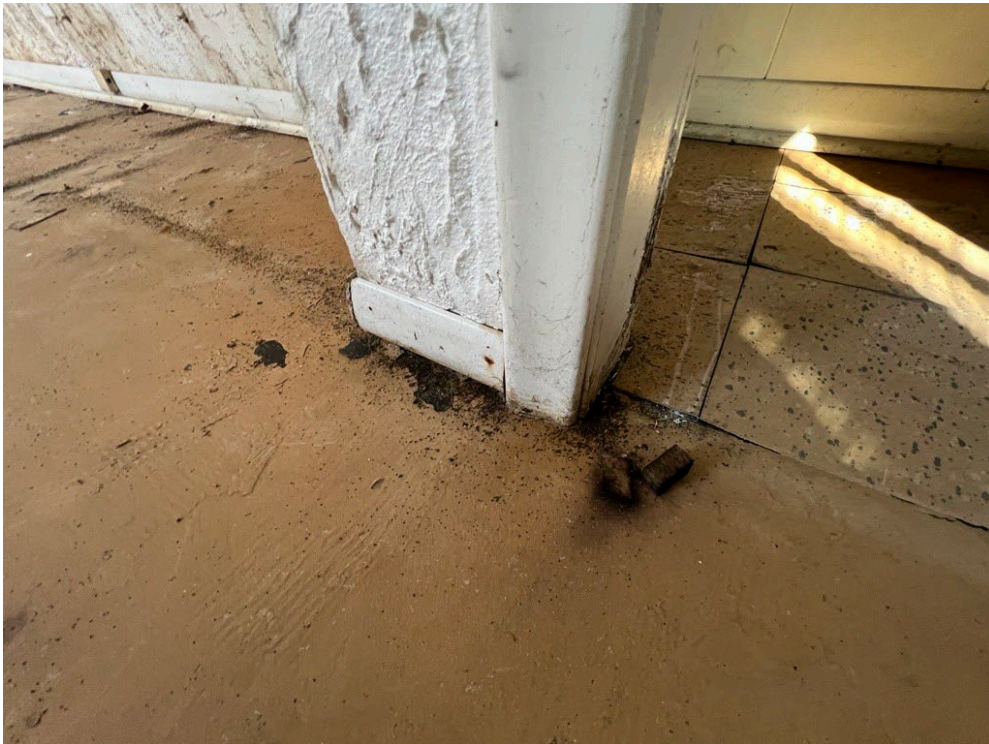
BASEMENT FLOOR WATER DAMAGE
