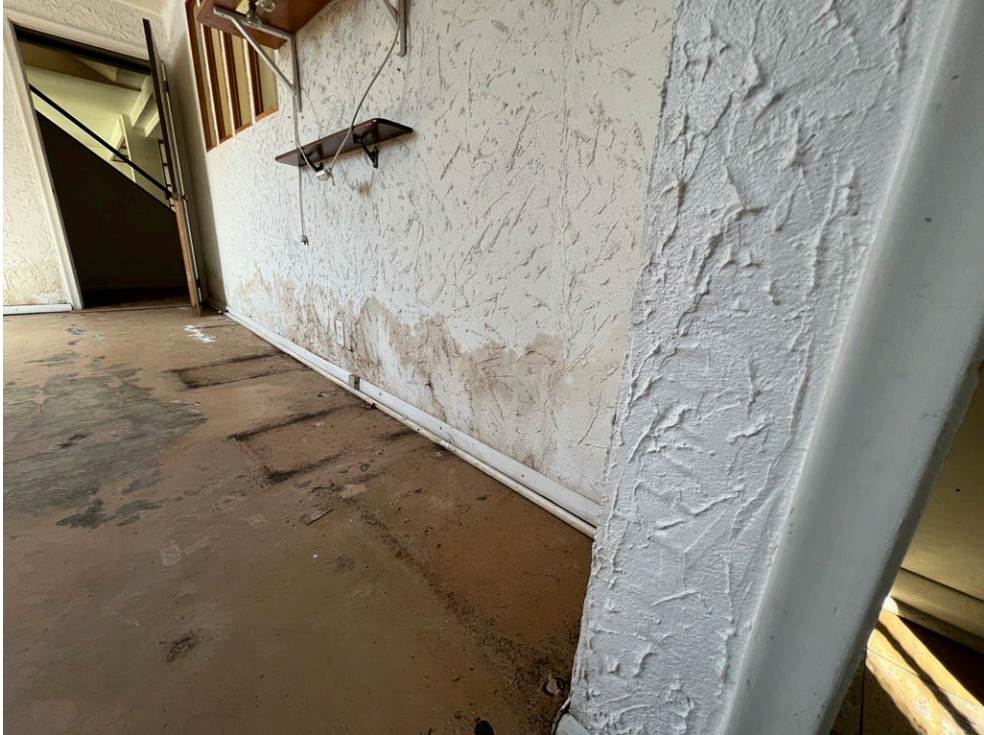
BASEMENT SHOWING WATER STAINING, MOULD
