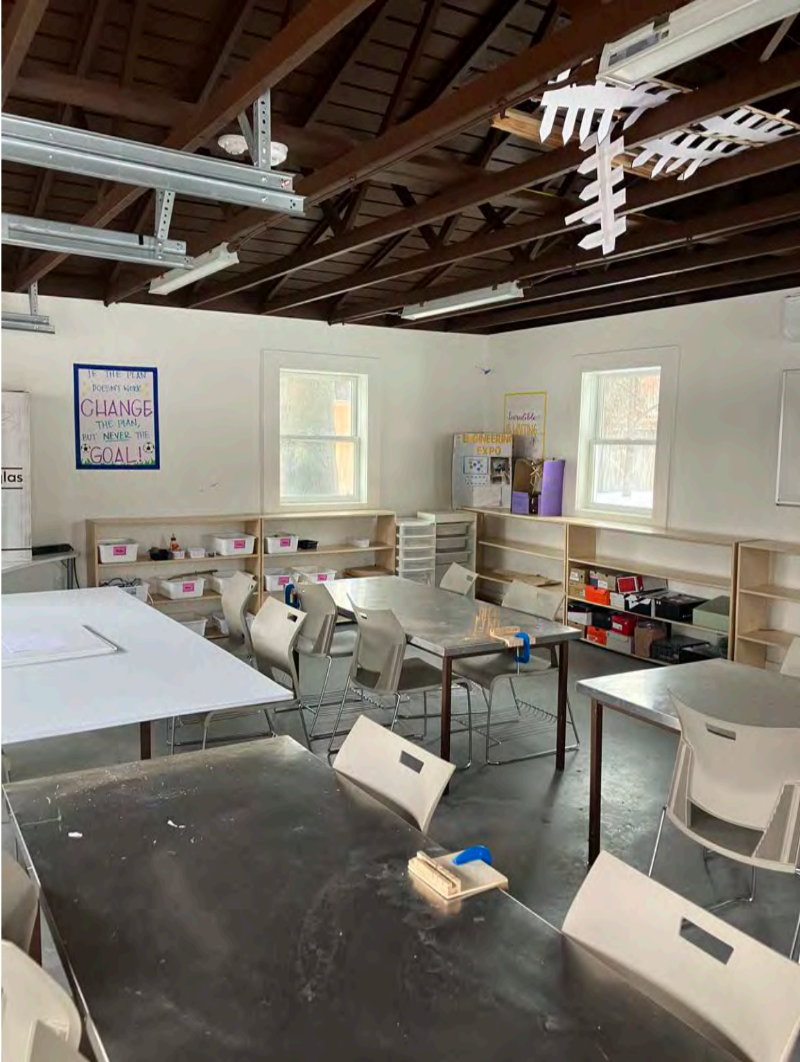
GARAGE – TO BE DEMOLISHED - a modern structure that has no cultural heritage value - concrete pad foundation – exposed roof rafters are modern dimensioned lumber – interior walls are drywall - date of construction estimated to be c.1970s or 1980s
