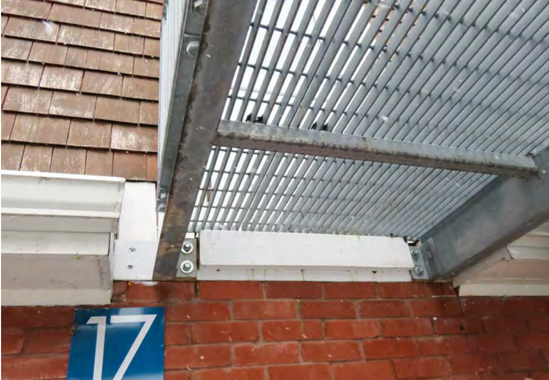
REAR ELEVATION – external fire exit stair from the 3 rd floor is to be removed – it is bolted into the masonry
