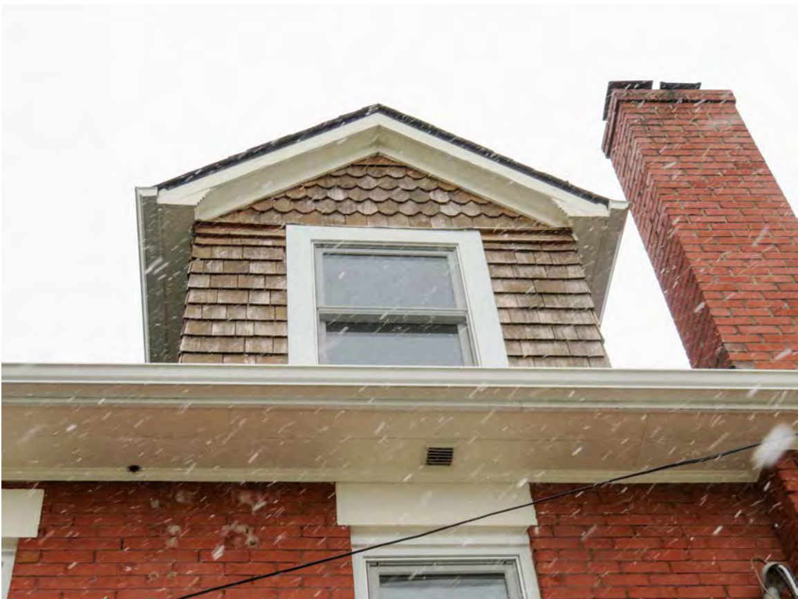
ROOF DORMER & BRICK CHIMNEY – the roof has a wide overhang – the wood shingles on the dormer are not original
