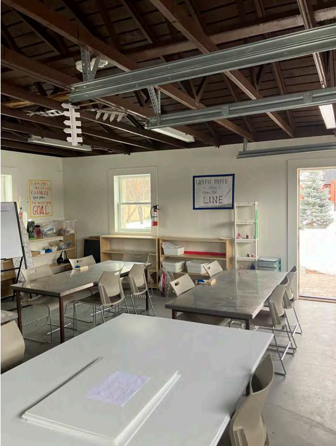
GARAGE – TO BE DEMOLISHED - a modern structure that has no cultural heritage value - concrete pad foundation – exposed roof rafters are modern dimensioned lumber – interior walls are drywall - date of construction estimated to be c.1970s or 1980s
